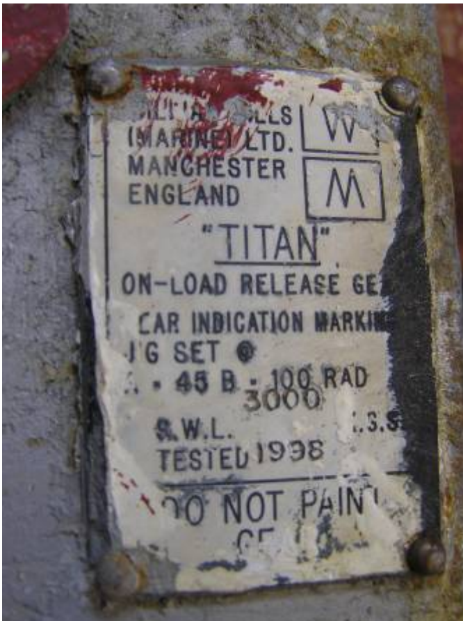
Figure 2: Manufacturer - Sign Plate of aft hoisting hook
