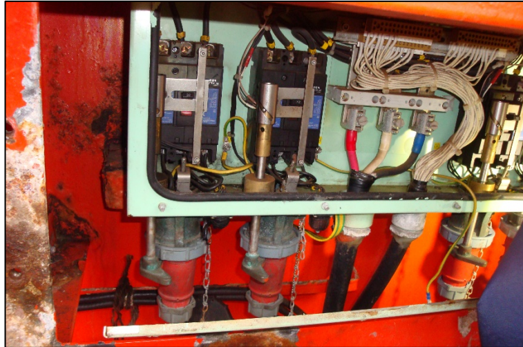
Figure 18: Slots with open distribution box 21
