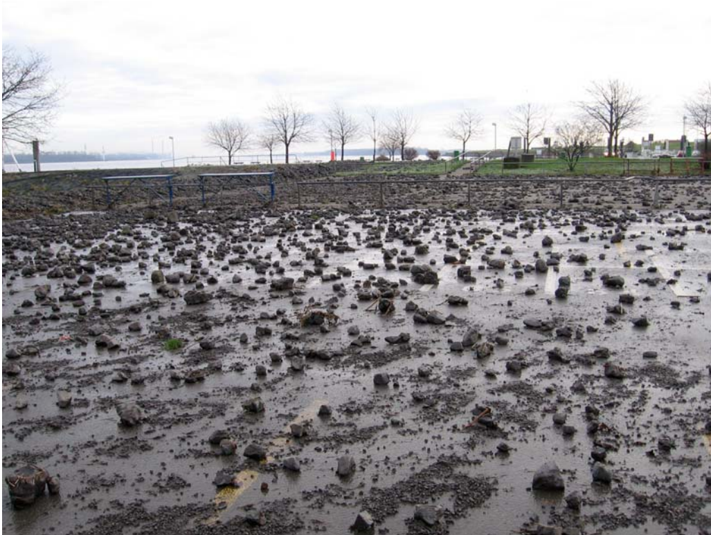
Swell damage to the Lühe quay on the Lower Elbe at Stade
