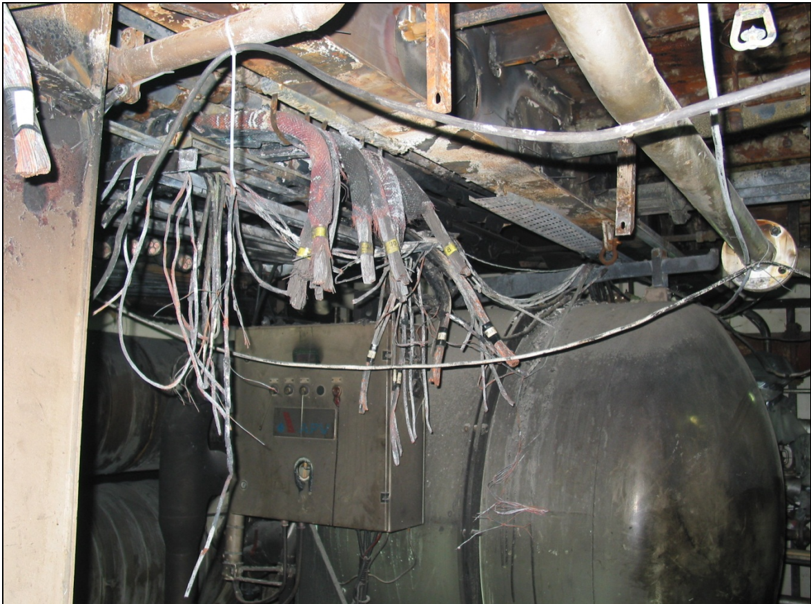
Fire in the engine room of the cruise ship DEUTSCHLAND, BSU Investigation Report Ref.: 216/10, published on 15/07/2011 Source: BSU
