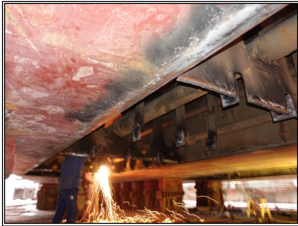
Damage to the bottom
