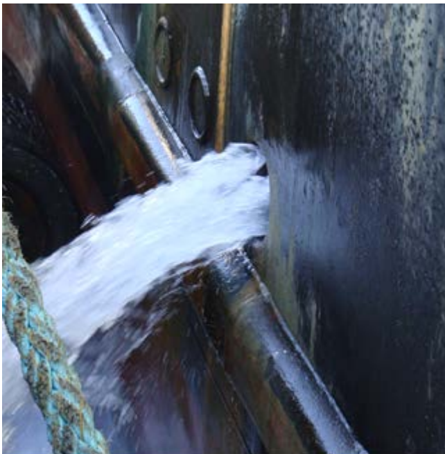
The open cooling water outlet of the JAN MARIA (source: BSU)
