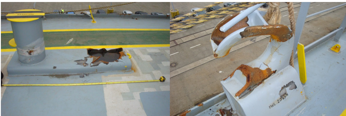
Ripped out bollards and destroyed fairlead on board the GLORY AMSTERDAM (source: BSU)
