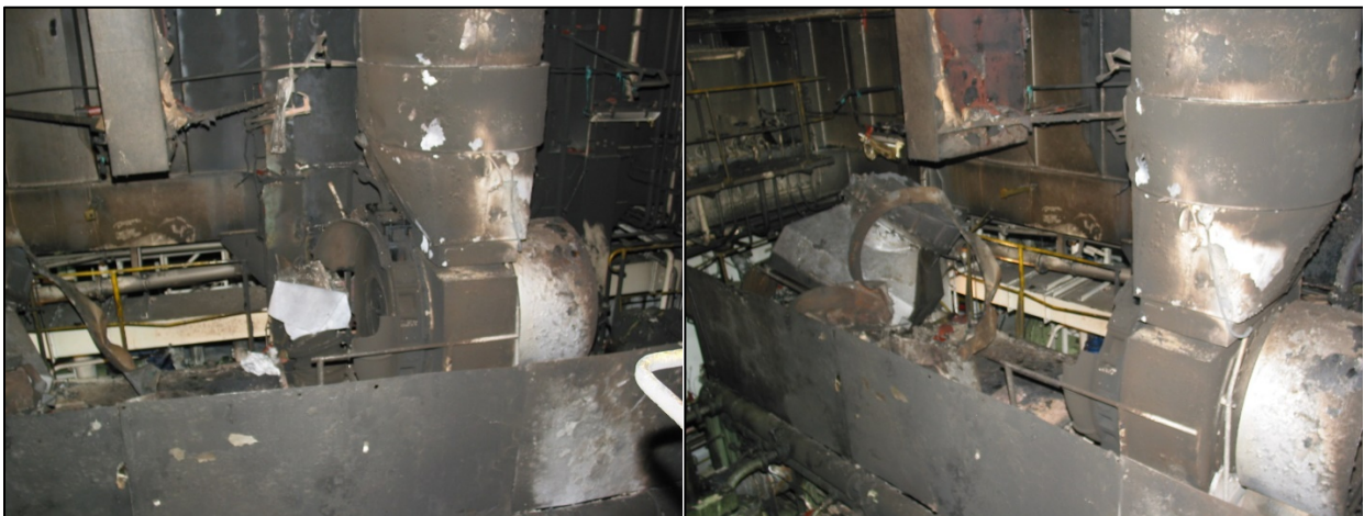
The engine room after the fire. Signs of destruction on the turbocharger are clearly visible. Source: BSU
