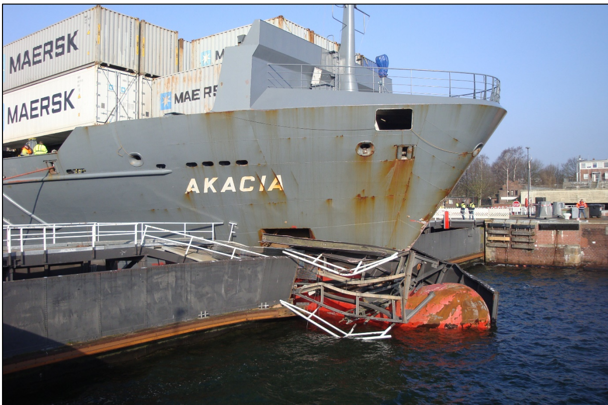
The bow of the ship penetrated the lock gate and settled on top of it. Source: BSU
