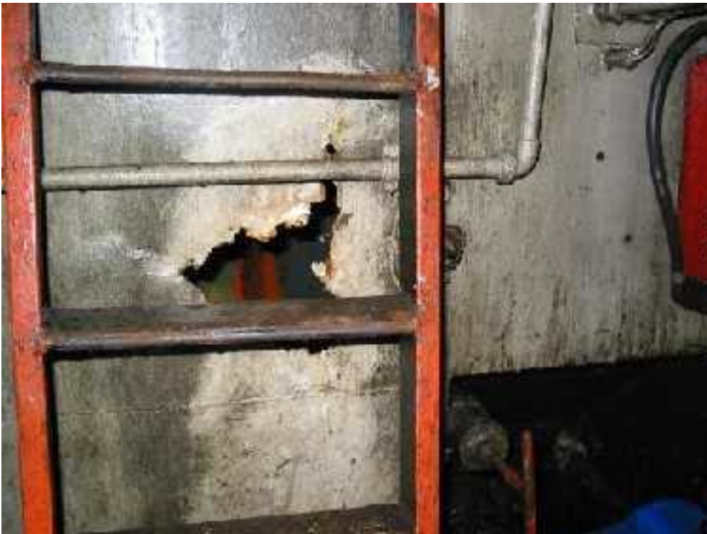
Photo 7, Engine room starboard astern
