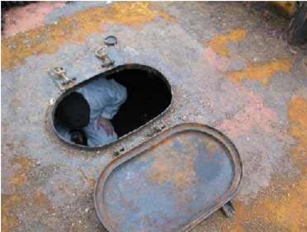
Photo 2, Manhole after peak
