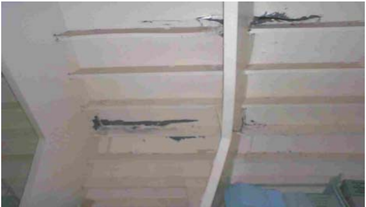
Picture 15: damage photo 11
