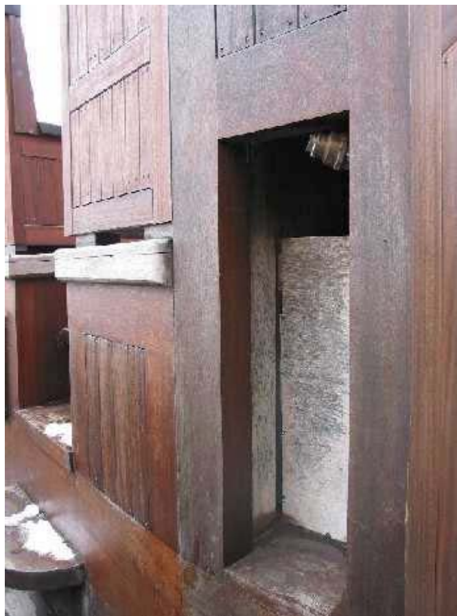
Photo 13, Starboard ventilation shaft (OUNV4P)
