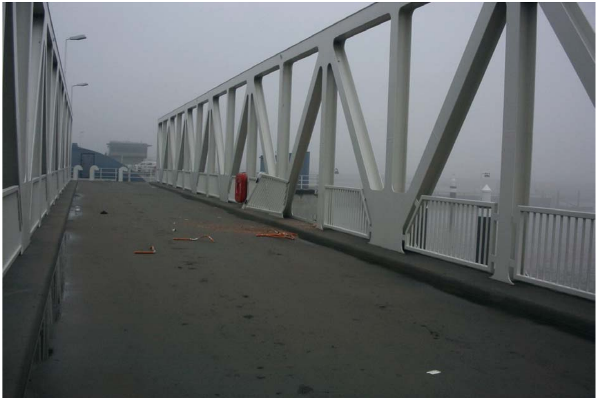
Figure 6: Damage at the flood barrage
