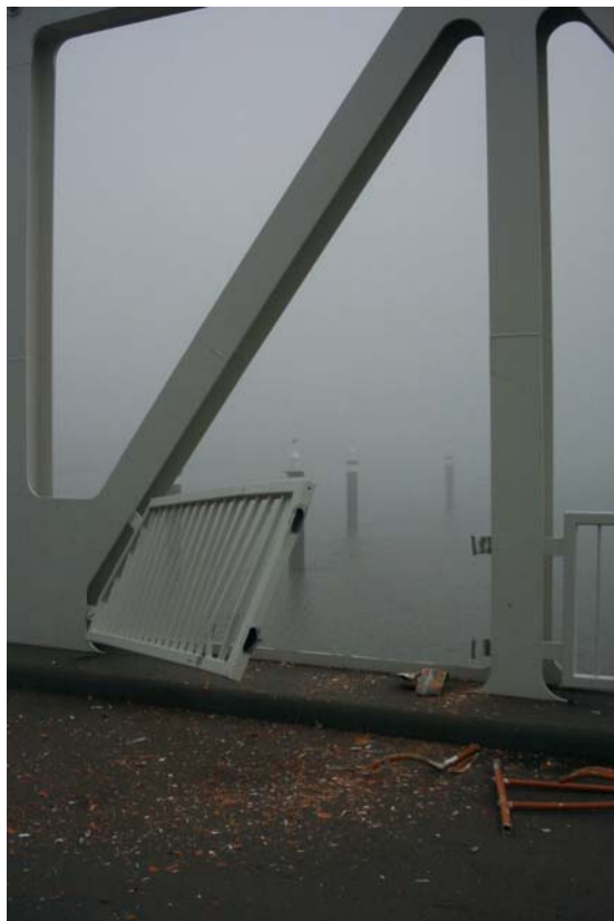
Figure 7: Detailed damage at the flood barrage
