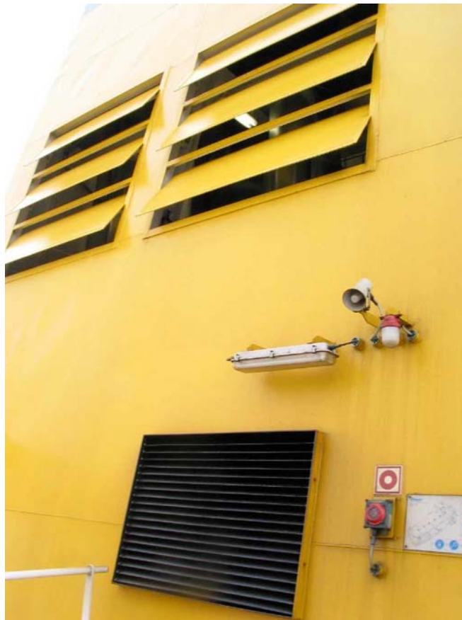
Figure 12: I.G. outlet and louver
