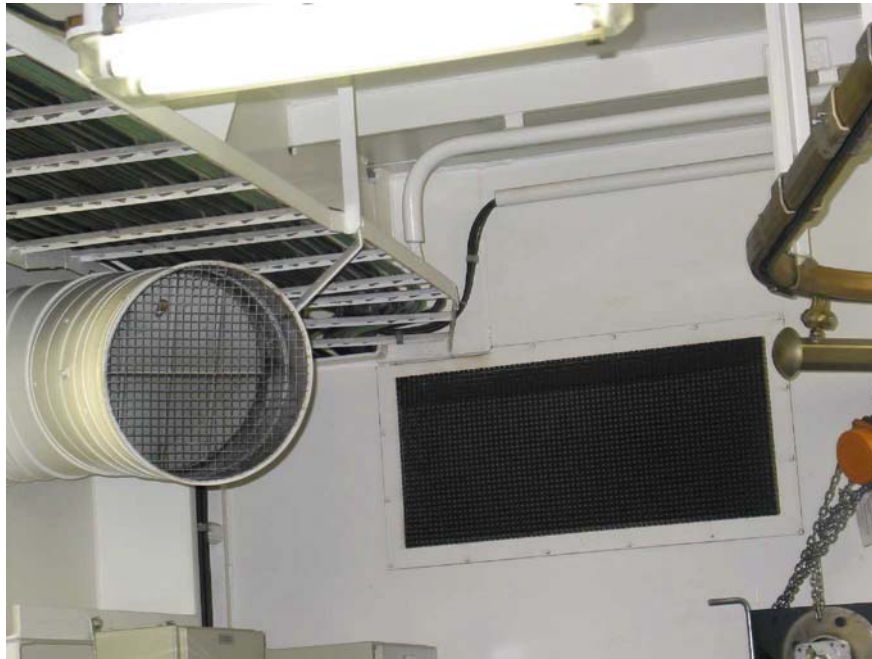
Figure 7: Ventilator separator room
