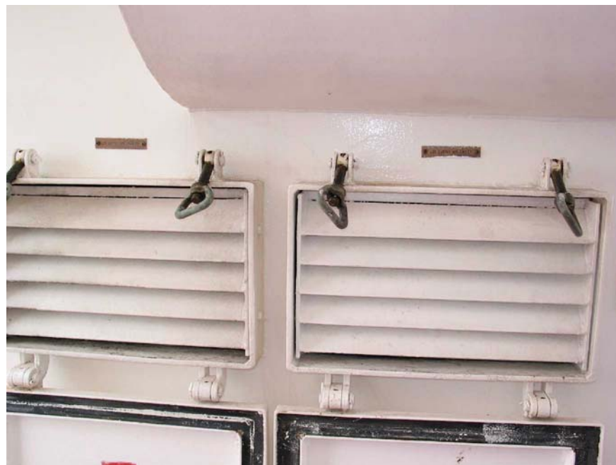
Figure 16: Air inlet, galley
