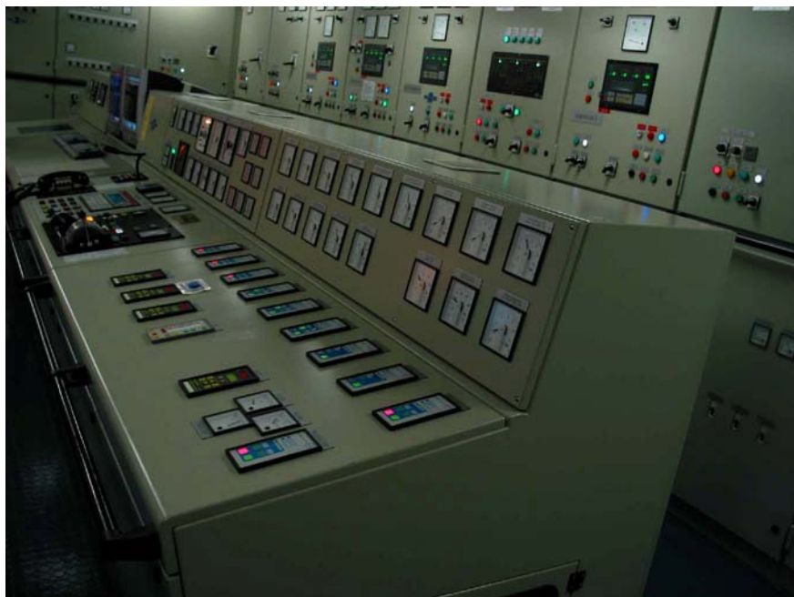
Figure 4: Engine control room
