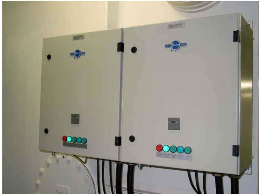
Figure 13: Switch cabinet engine room ventilator
