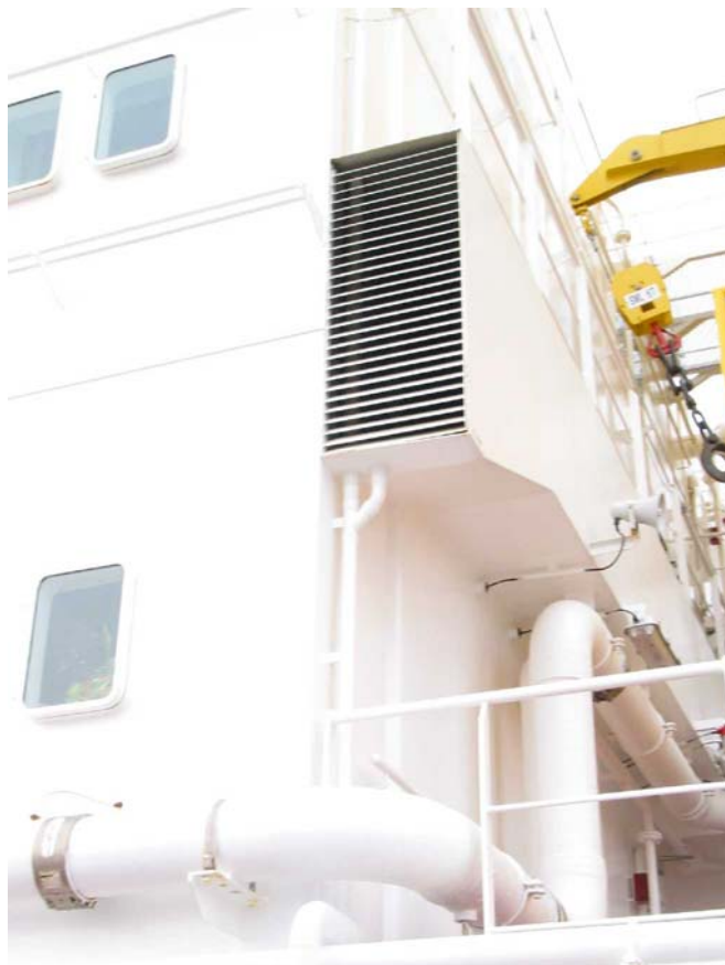
Figure 15: Air inlet air conditioner, provisions room with I.G. line running beneath
