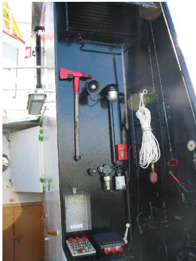
Figure 5: Control console, Towing winch
