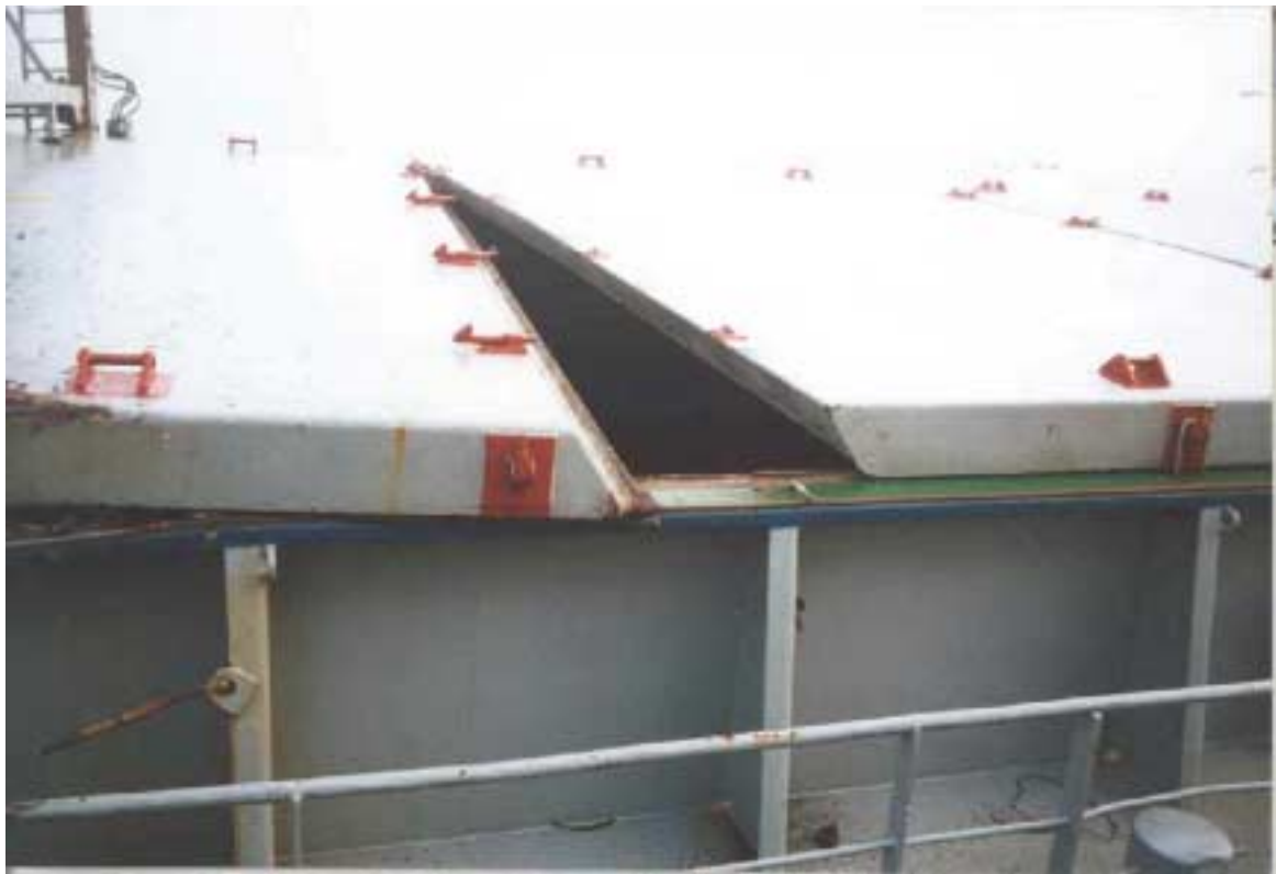
Figure 8: Photo of damage 2
