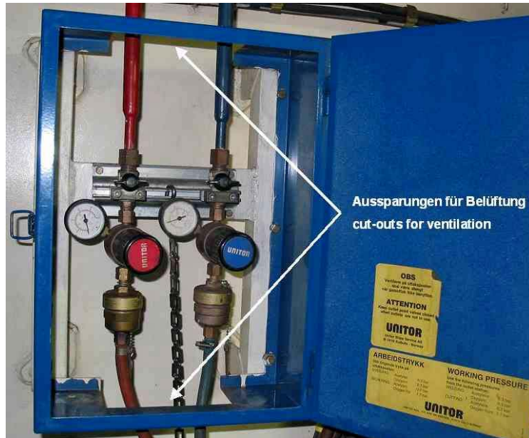
Figure 11: Fitting cabinet ventilated in accordance with regulations
