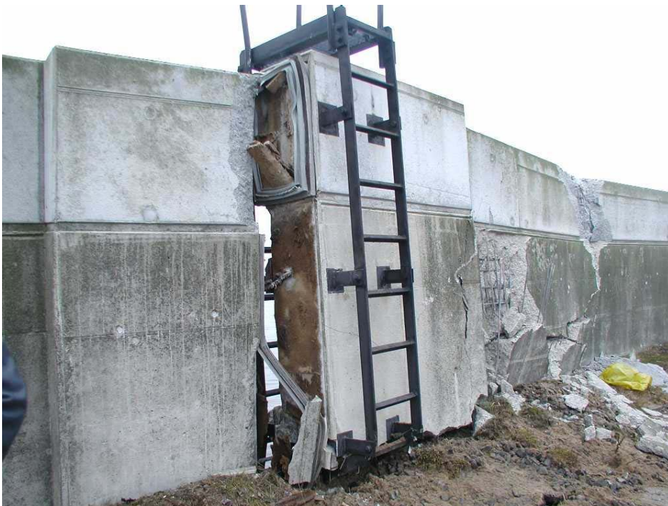
Figure 19: Photo of the damage 5 - Köhlbrandhöft/sheet piling
