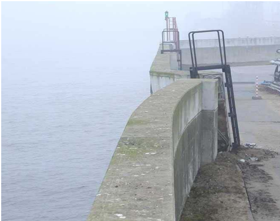
Figure 18: Photo of the damage 4 - Köhlbrandhöft
