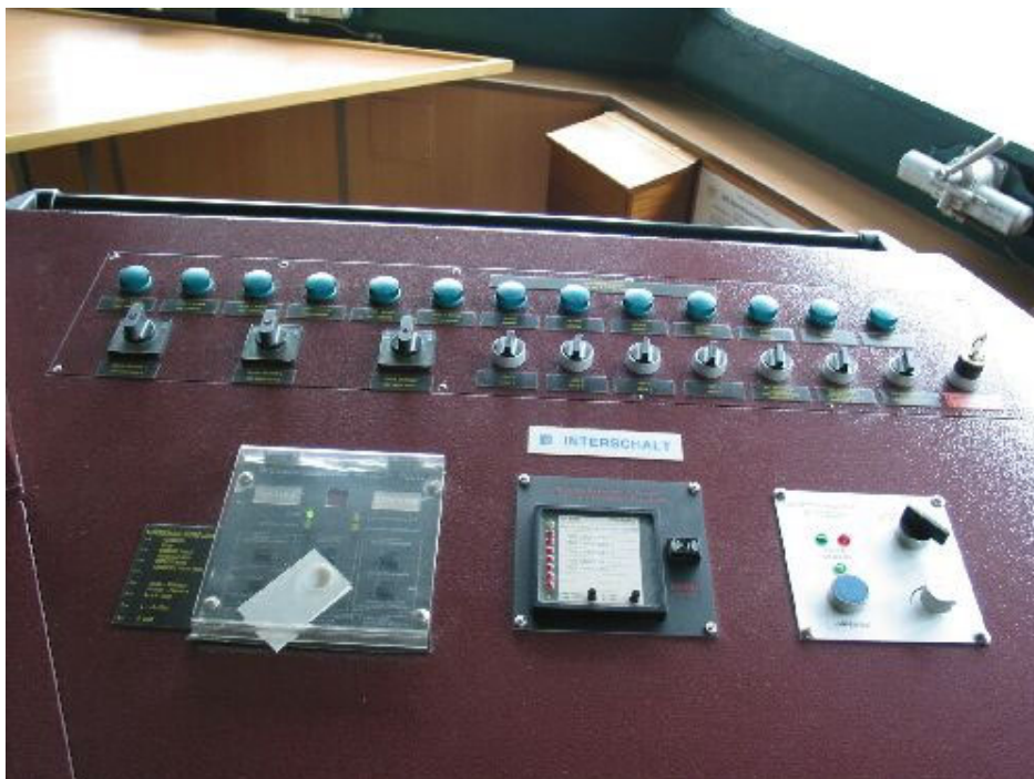
Figure 7, Switch consol deck and hatch lighting
