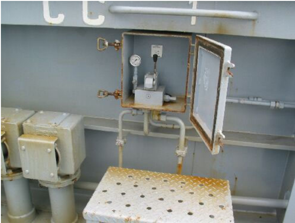
Figure 8, Hatch controller Hatch 1
