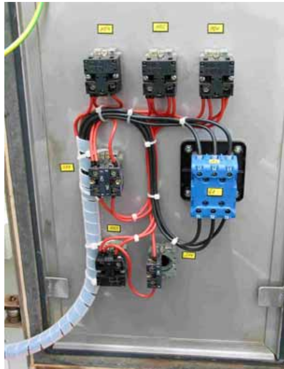
Figure 18: Inside of switch cabinet door
