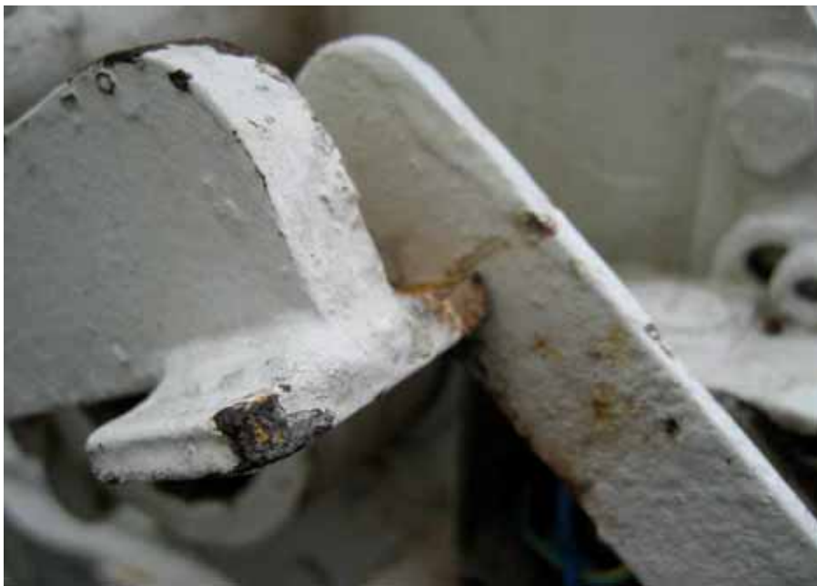
Figure 19: Limit switch lever behind the safety bar
