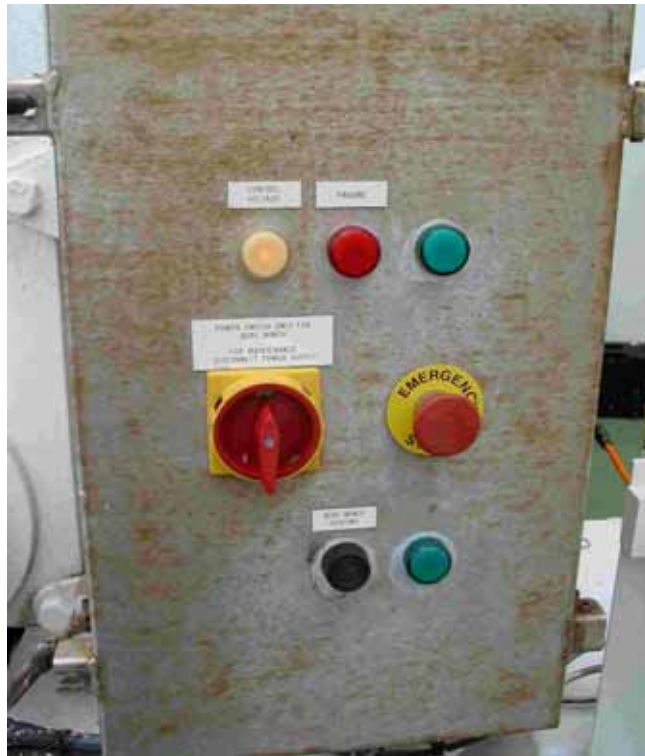
Figure 4: Switch cabinet; winch motor operating elements
