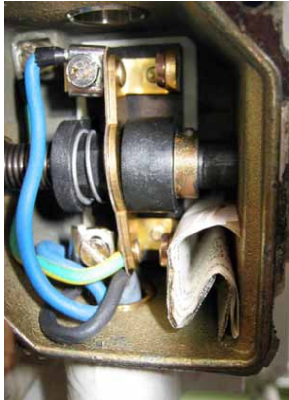
Figure 16: View of interior of limit switch
