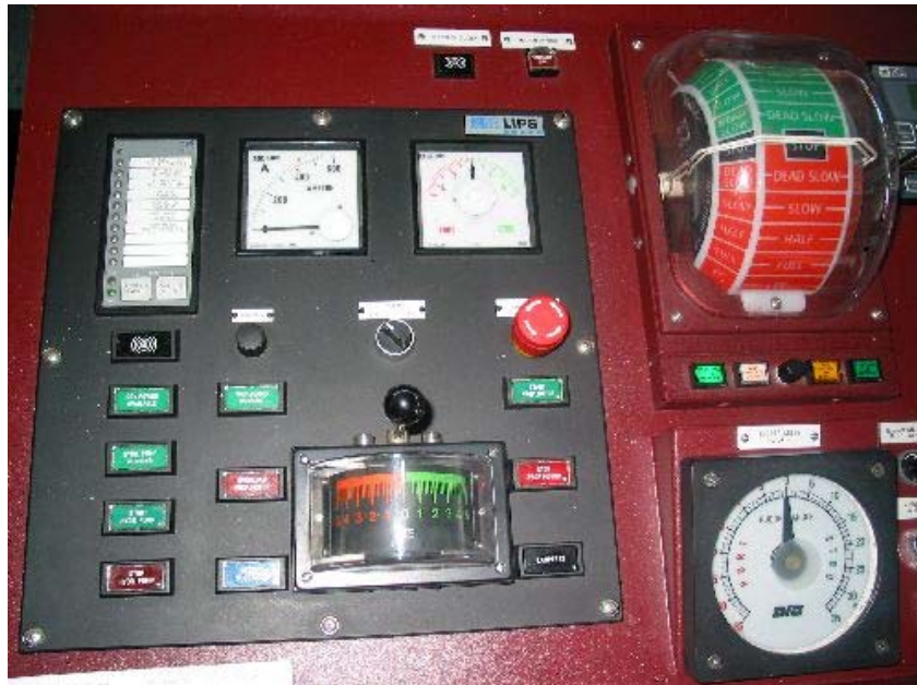
Figure 6: Control console bridge
