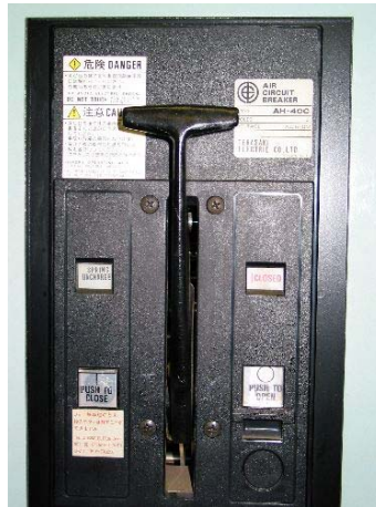
Figure 9: Main switch bow thruster
