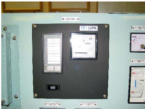
Figure 7: Control console engine control room
