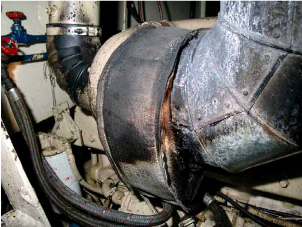
Figure 13: Exhaust gas turbocharger insulation
