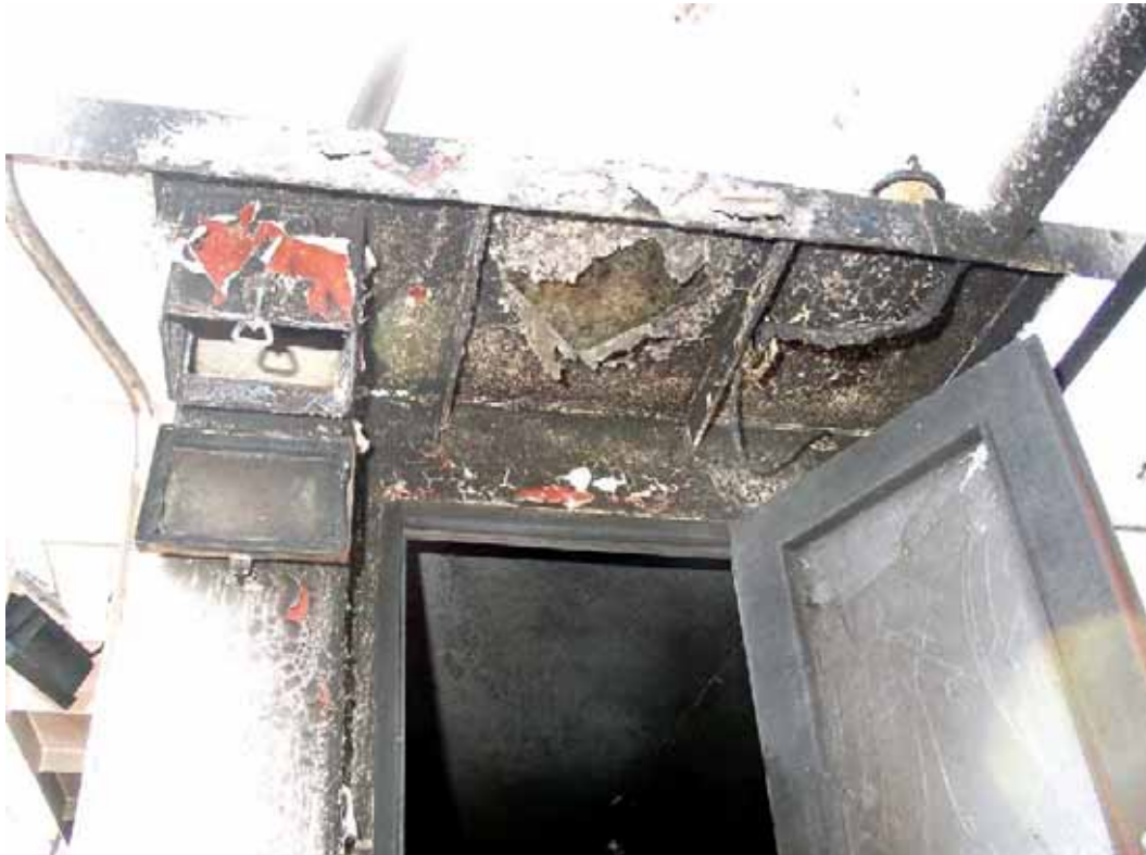
Figure 4: Galley door aft
