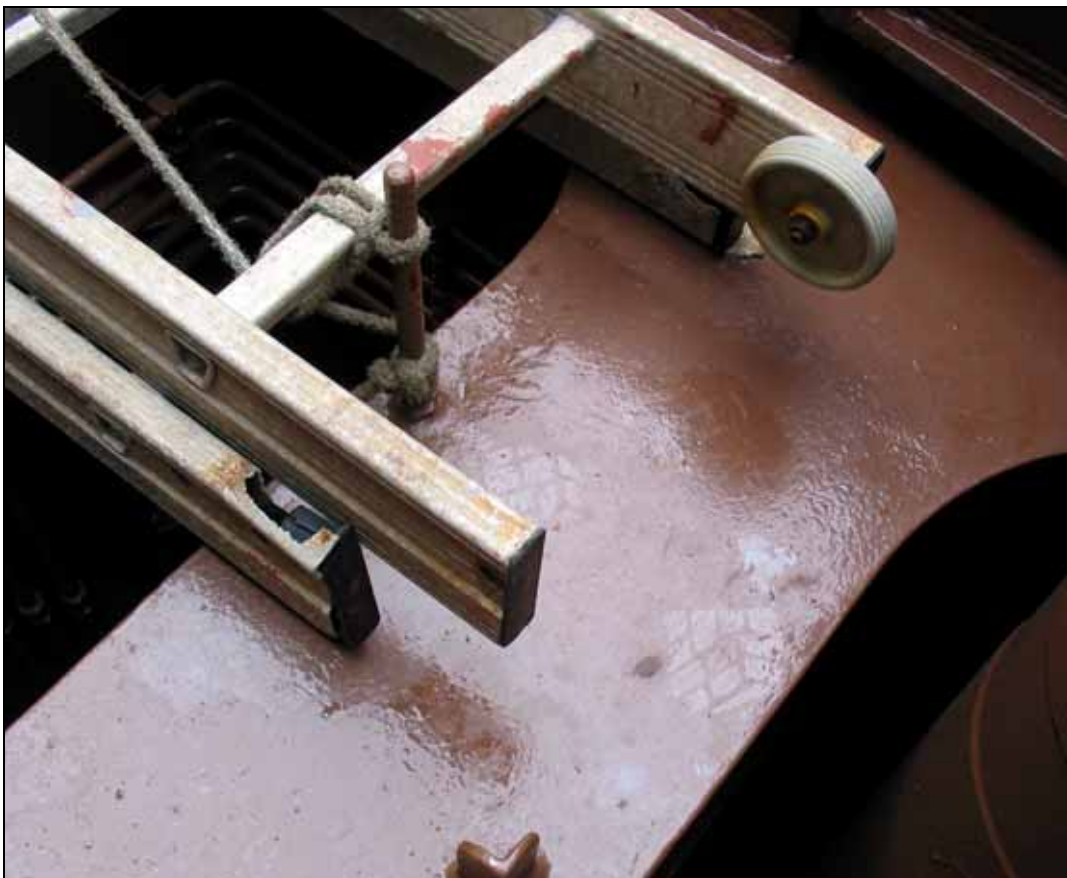
Figure 12: Corrosion and missing roller
