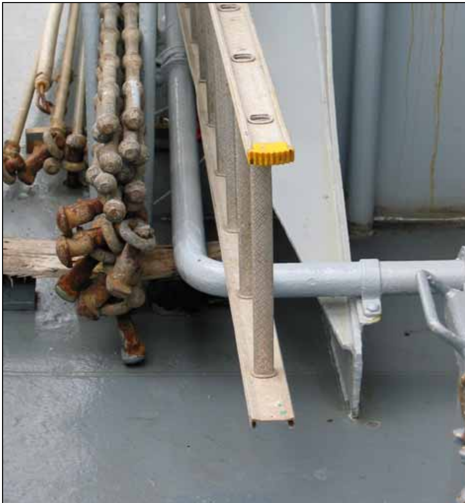
Figure 10: Missing rubber foot
