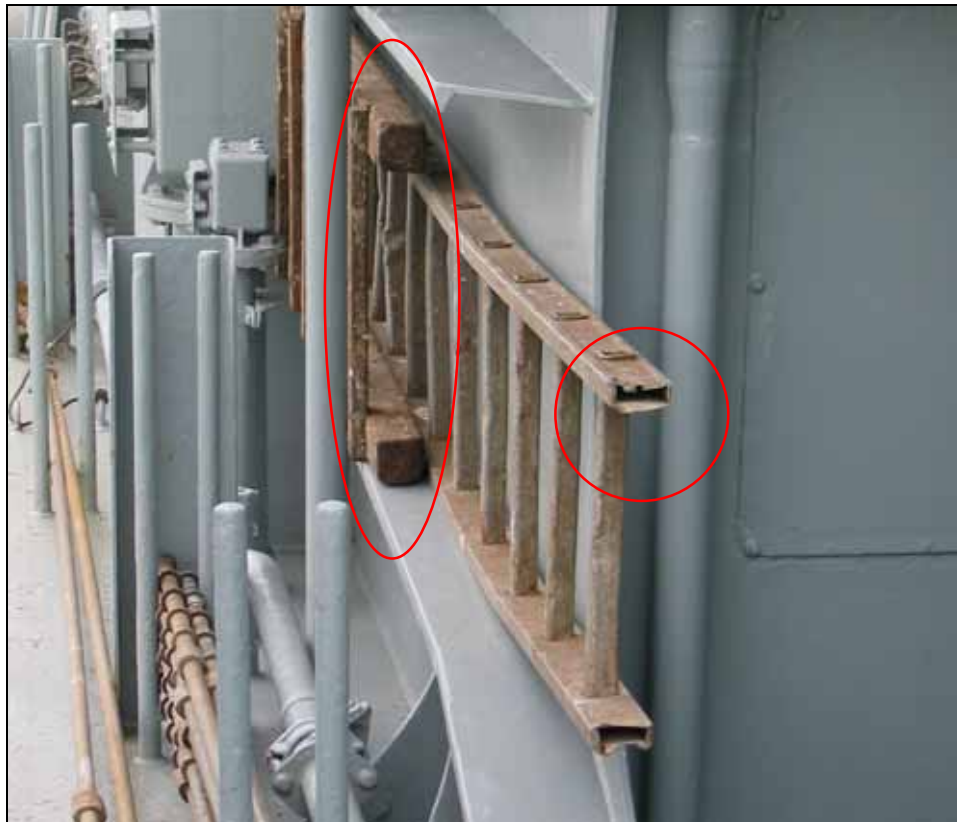
Figure 14: Damaged aluminium ladder, wooden ladder with rungs nailed on
