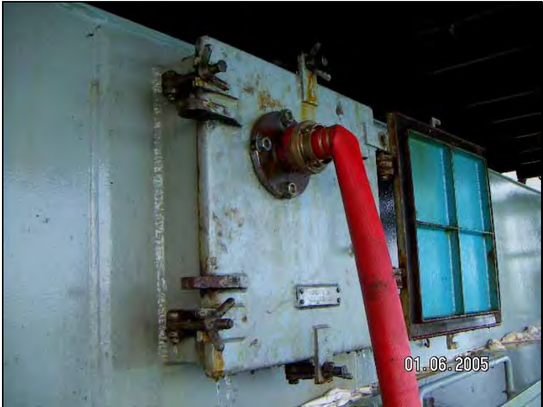
Figure 3: Ventilator damper converted for cooling
