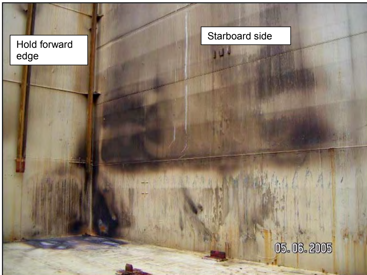
Figure 5: Hold 6 - forward edge stbd.
