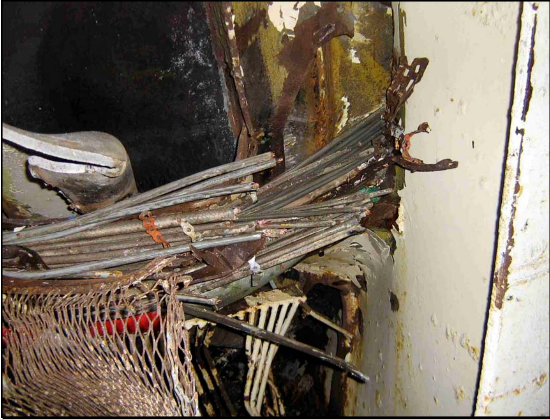
Fig. 7: TOR DANIA – damage photo 2
