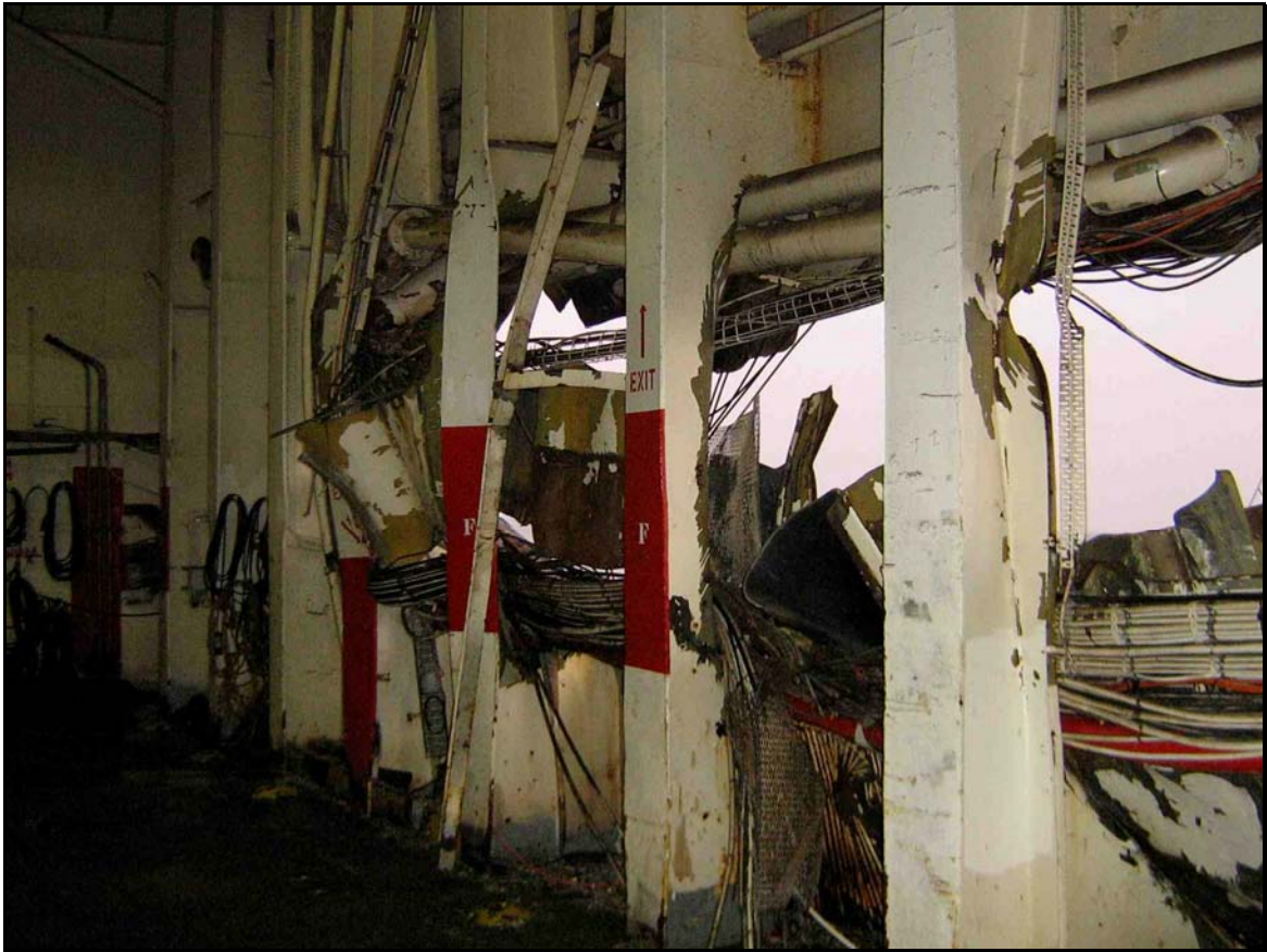
Fig. 6: TOR DANIA – damage photo 1
