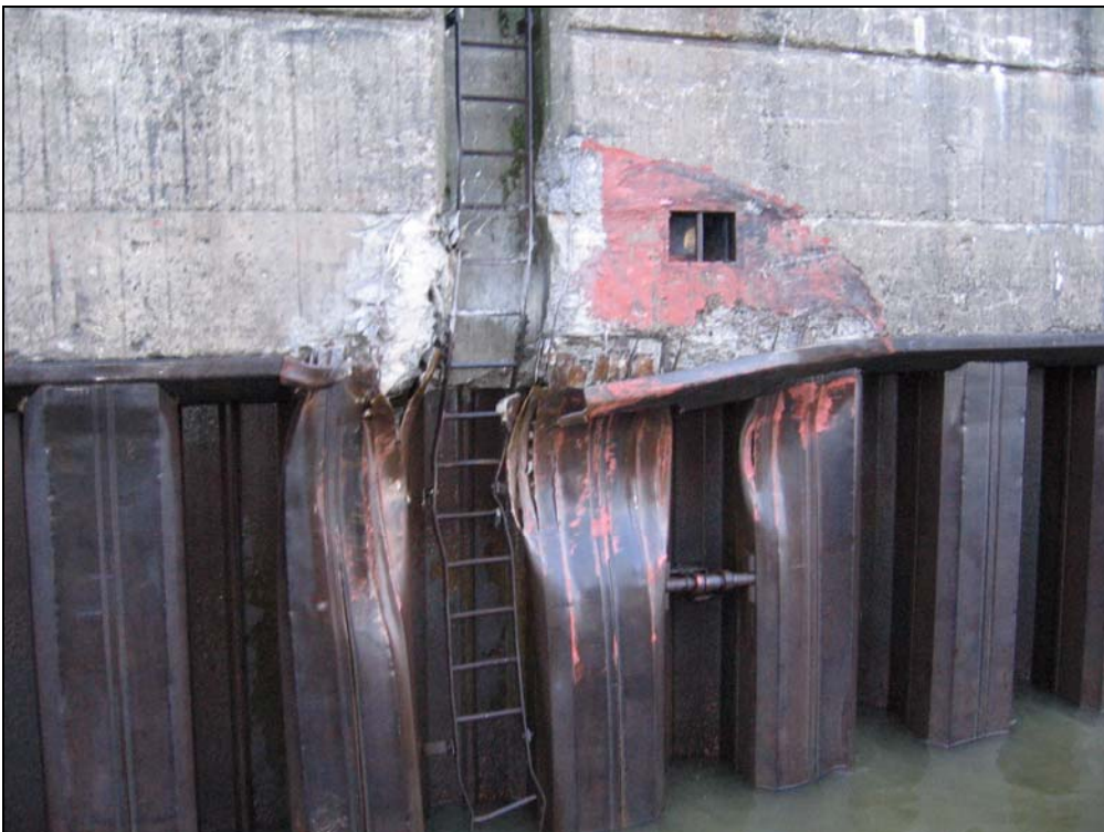
Figure 4: Close-up View of the Damaged Quay
