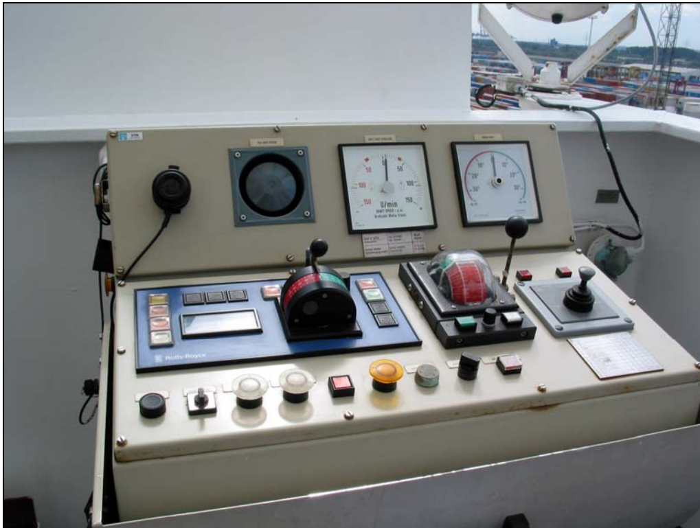
Figure 8: Secondary Control Position in the Starboard Wing of the Bridge
