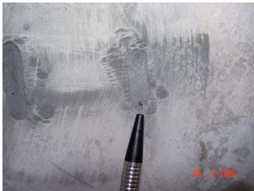
Fig. 6: Sites of previous repair work
