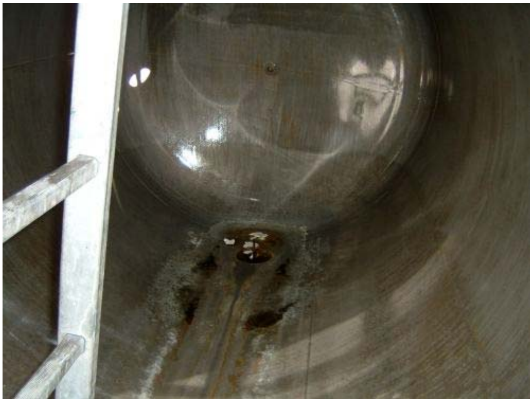
Fig. 14: View of the inside of the tank container
