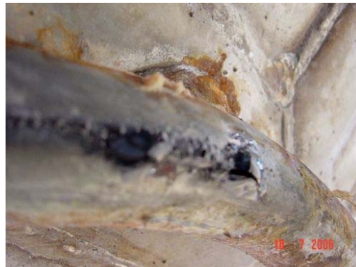
Fig. 7: Eroded pipe in the heating system
