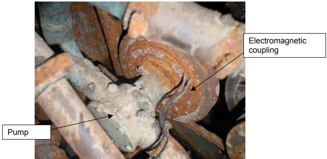
Figure 15: Main draining pump
