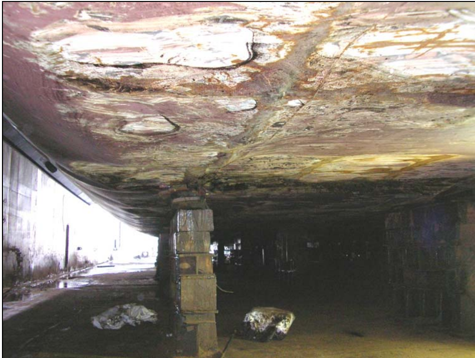
Fig. 5: Damages to the underwater hull 22
