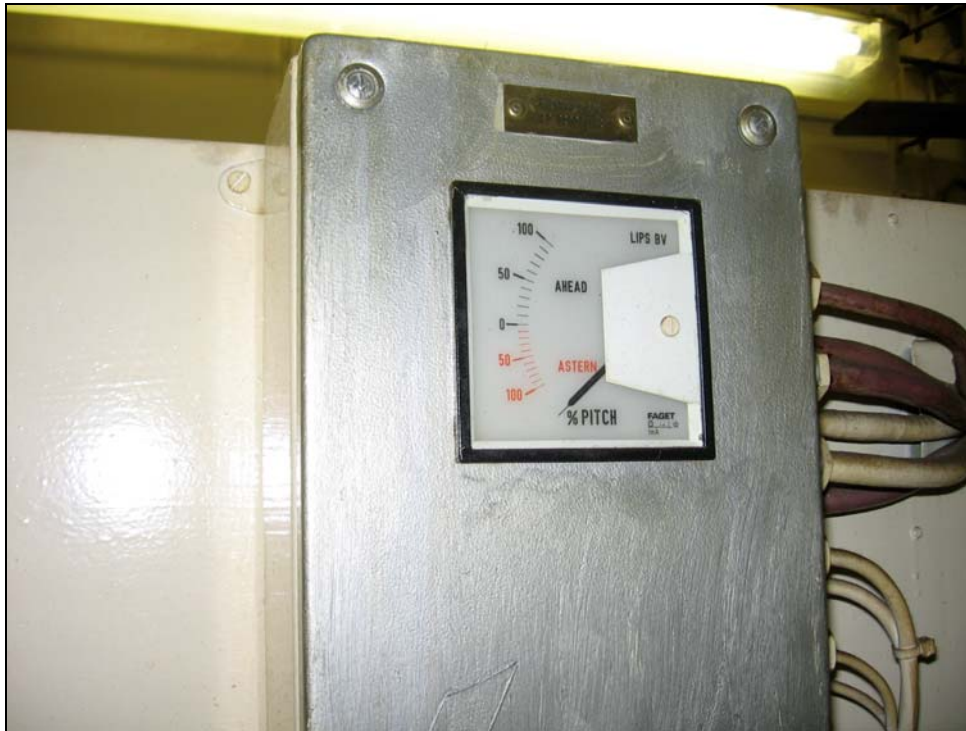
Figure 17: Pitch indicator in the engine room after the collision
