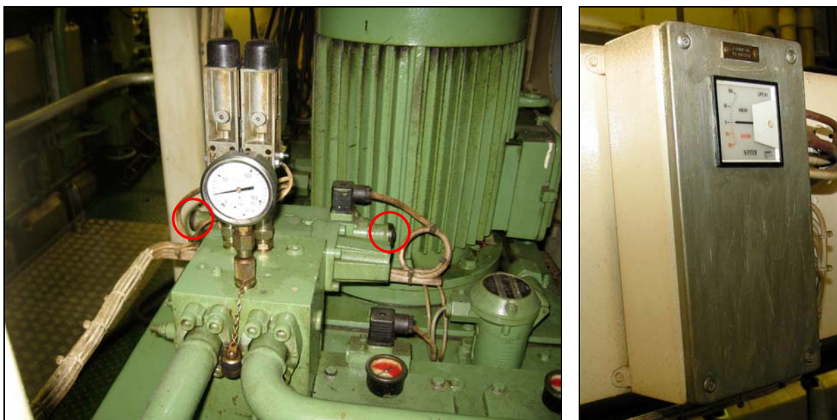
Figure 14: Pump station with pitch indicator placed above
