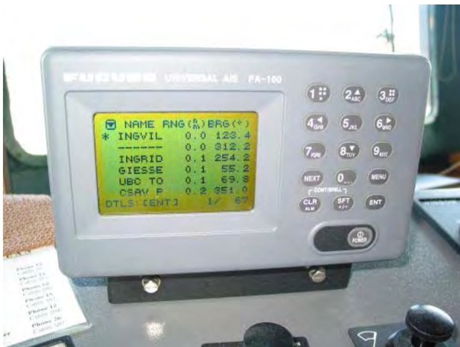
Fig. 7: AIS installation SVEN
