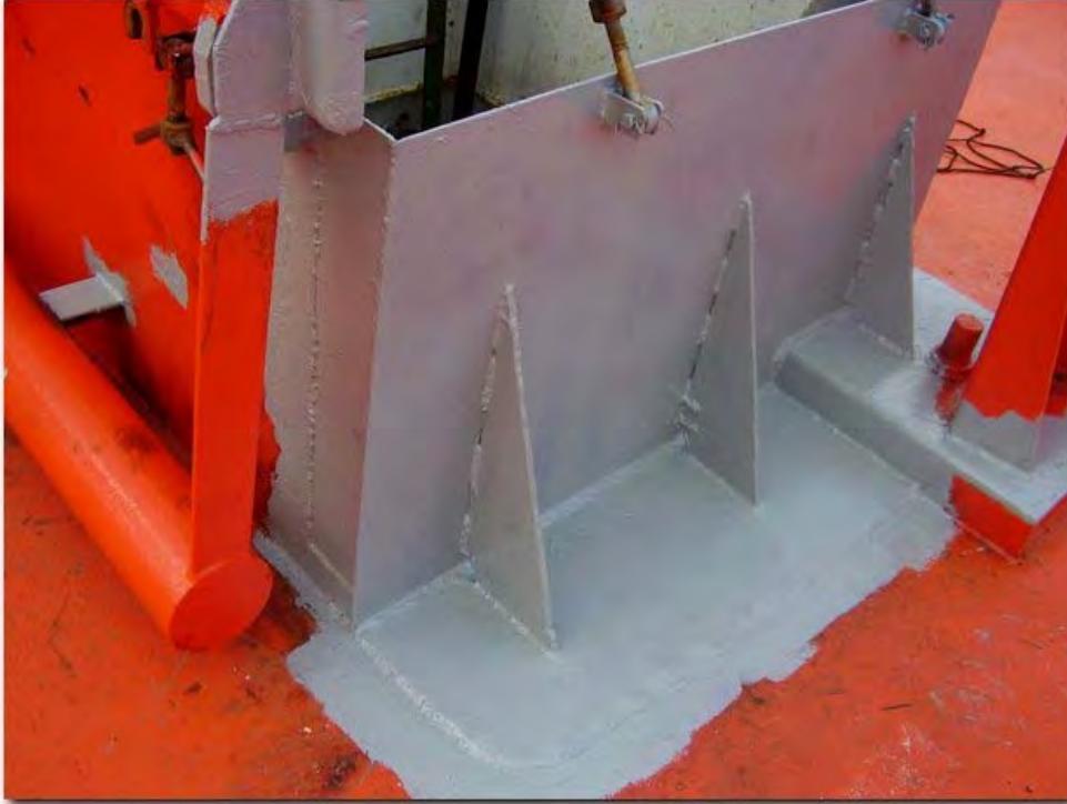
Figure 16: Repaired and reinforced hatch coaming on the forecastle of the CAP EGMONT
