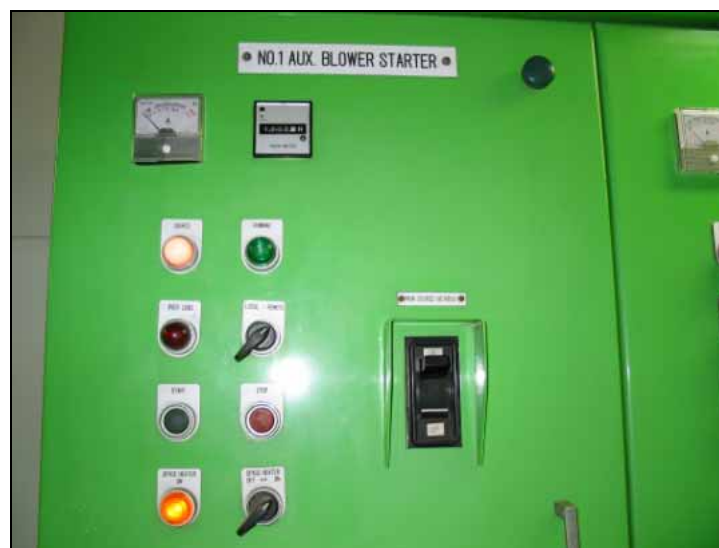
Figure 36: Main auxiliary fan panel – close-up view
