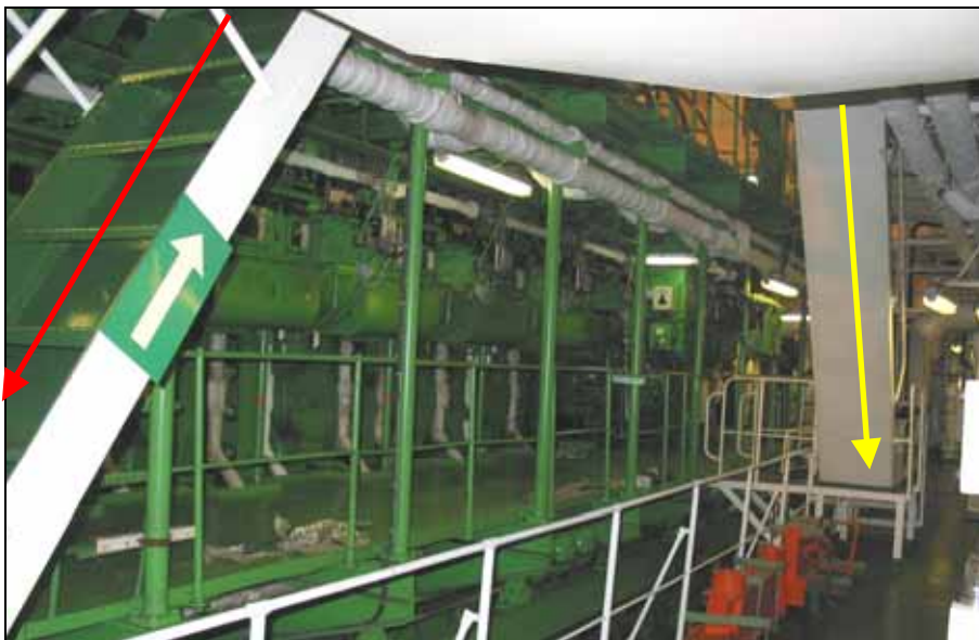
Figure 6: Companionways 1 and 2 from the cylinder head level to the scavenge air receiver level (2) 17
