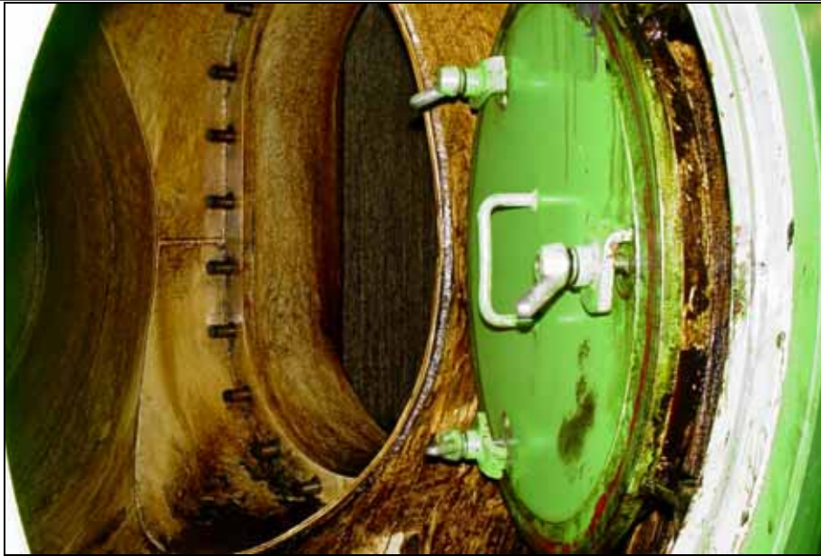
Figure 20: Scavenge air receiver man hole cover – forward end – swung inwards
