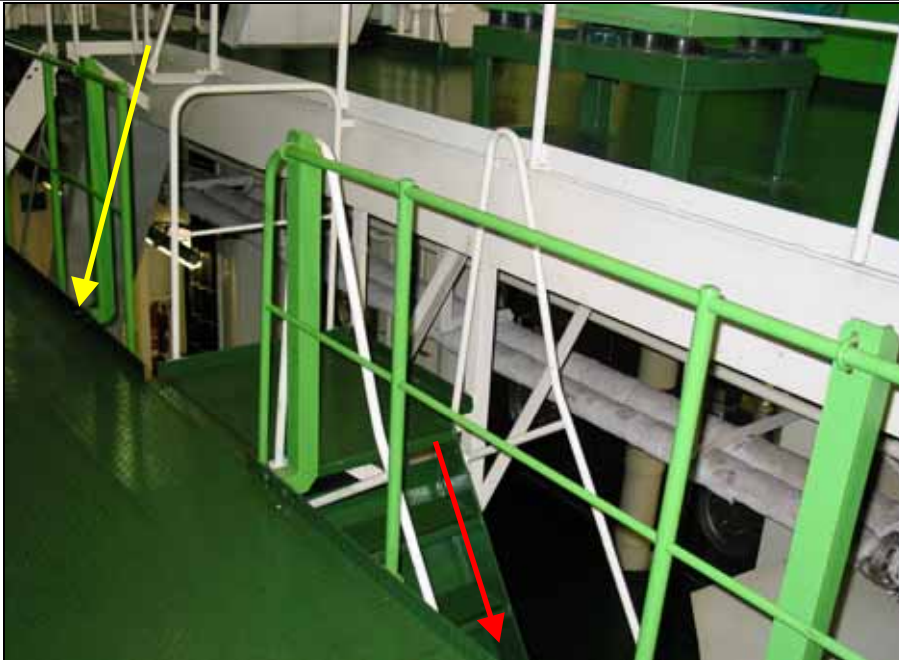
Figure 5: Companionways 1 and 2 from the cylinder head level to the scavenge air receiver level (1) 16
