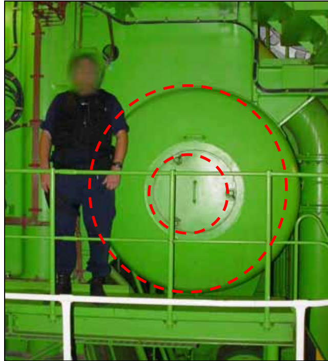
Figure 19: Scavenge air receiver – aft end with access hatch closed
