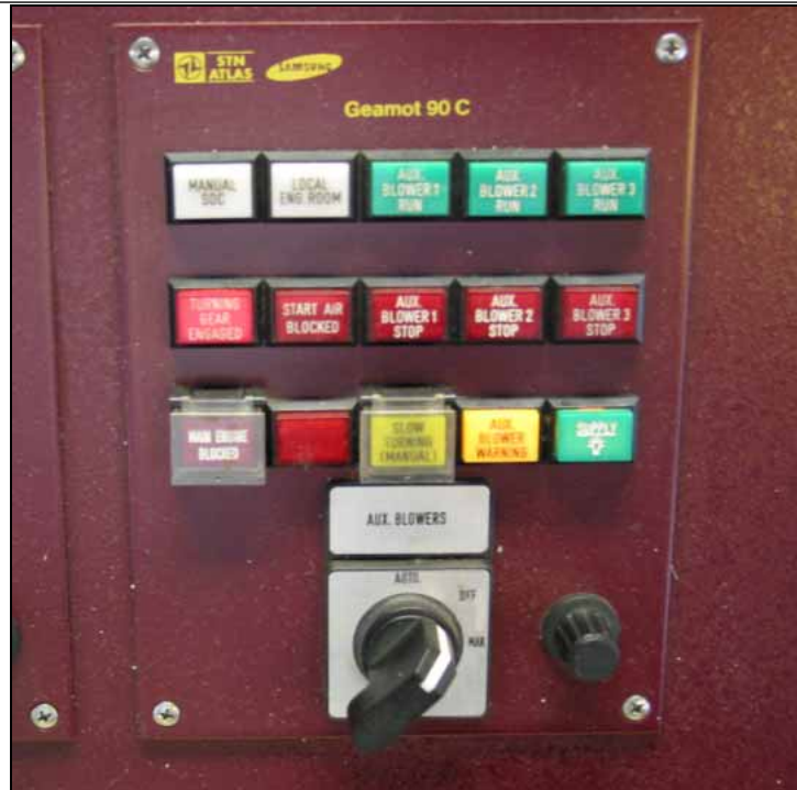
Figure 37: Auxiliary fan control panel on the bridge console
