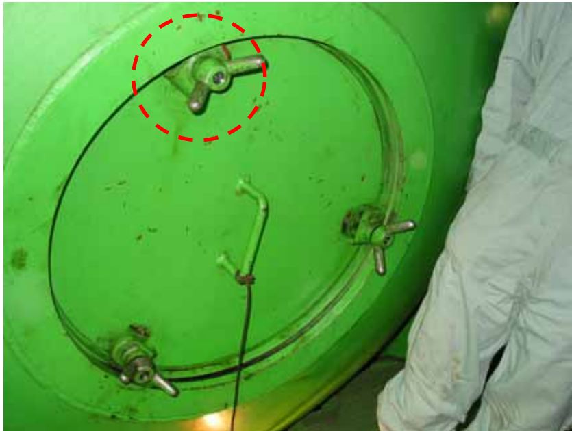
Figure 33: Partial locking condition – overall view
