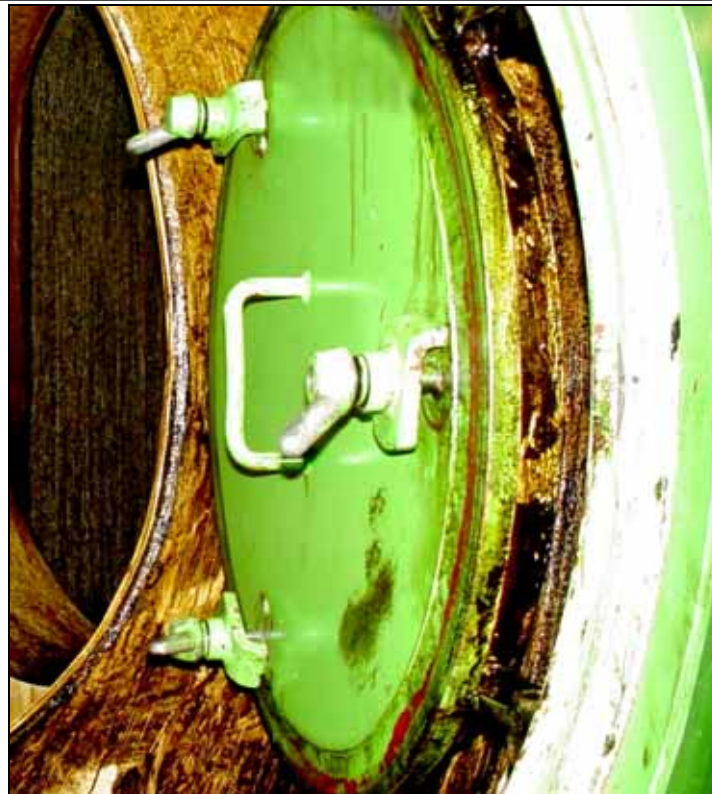
Figure 30: Bolts remain in the tangential opening position
