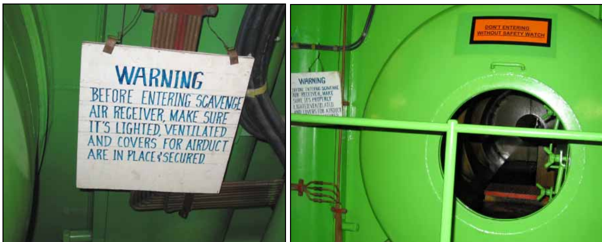
Figure 60: Warnings at the access hatch
