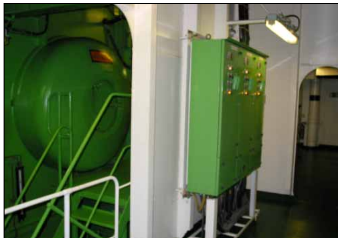
Figure 35: Main auxiliary fan panels 1 to 3
