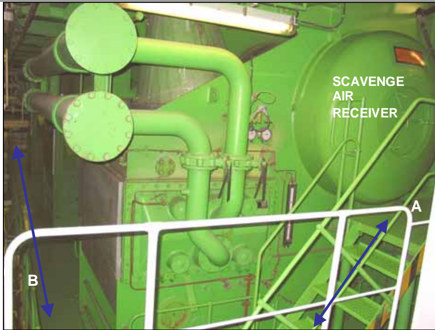
Figure 12: Scavenge air receiver level, forward end and starboard side 21
