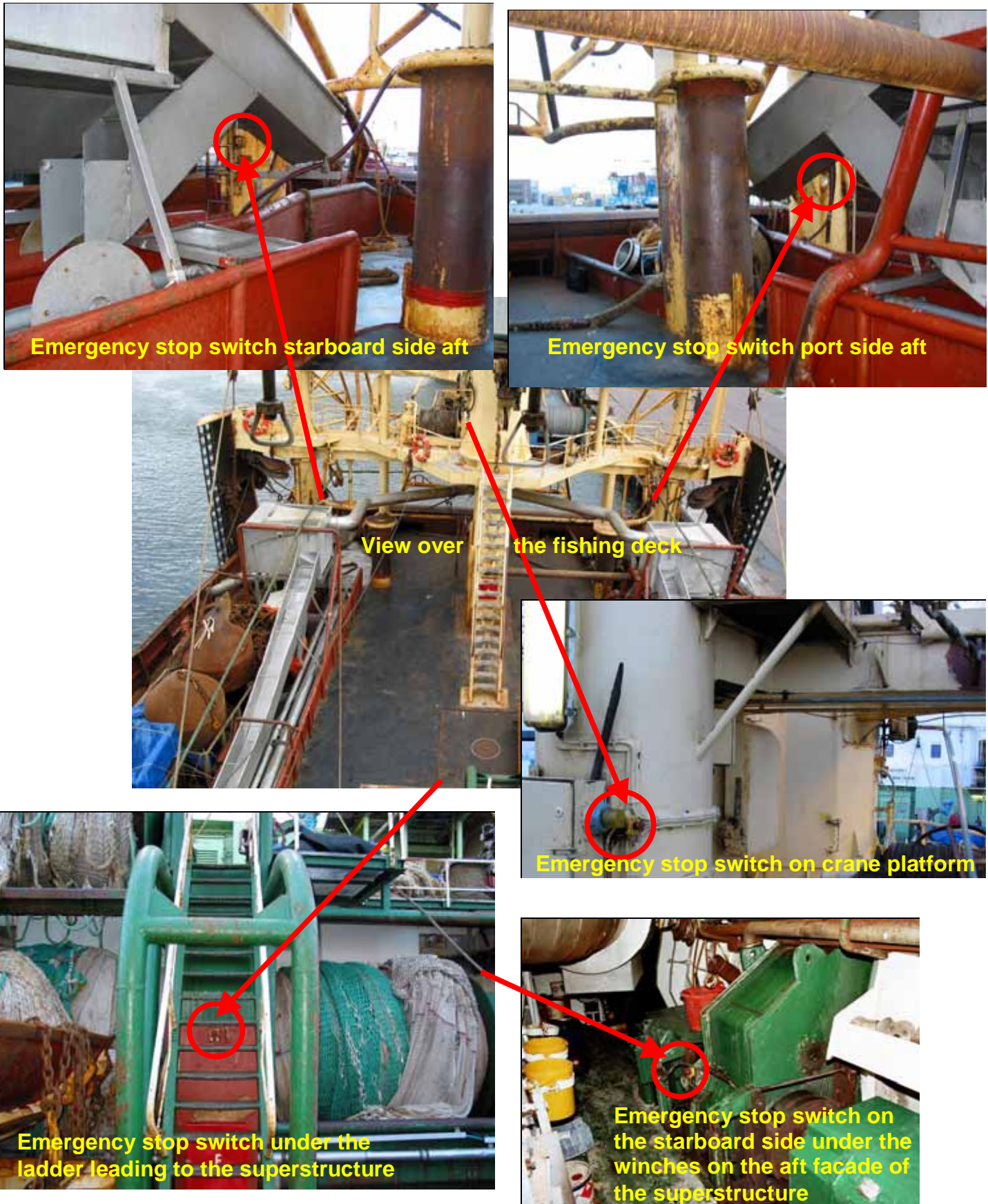
Figure 19 : Illustration of emergency stop switches on the fishing deck
