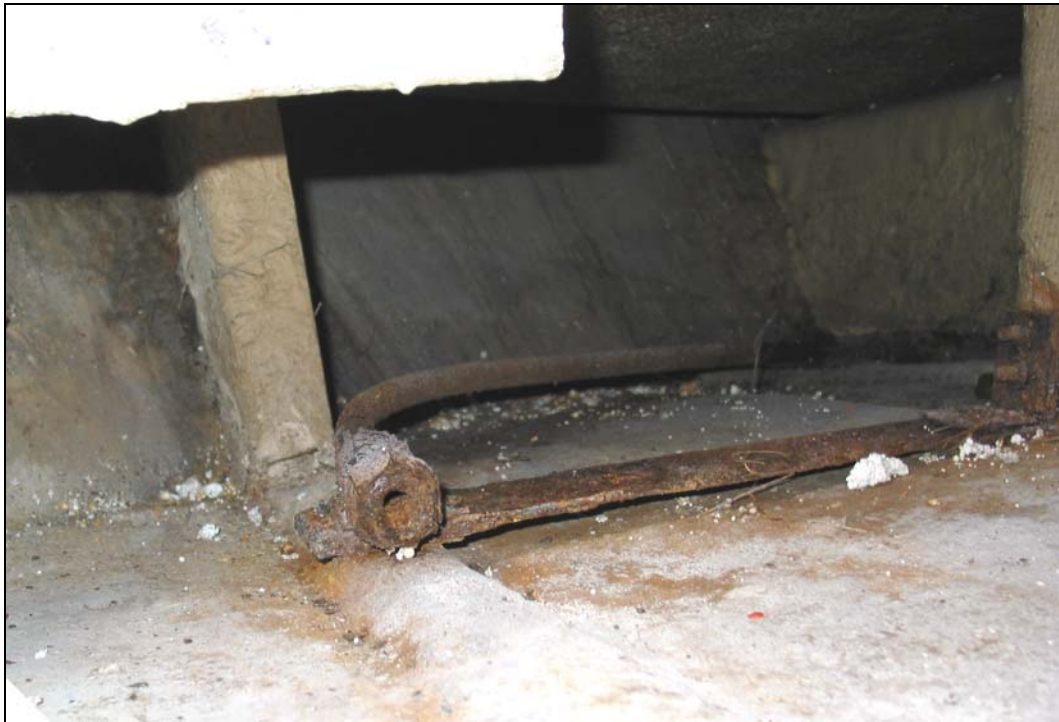
Figure 19: Guide tube for the starboard operating wire rope at the forward exit point
