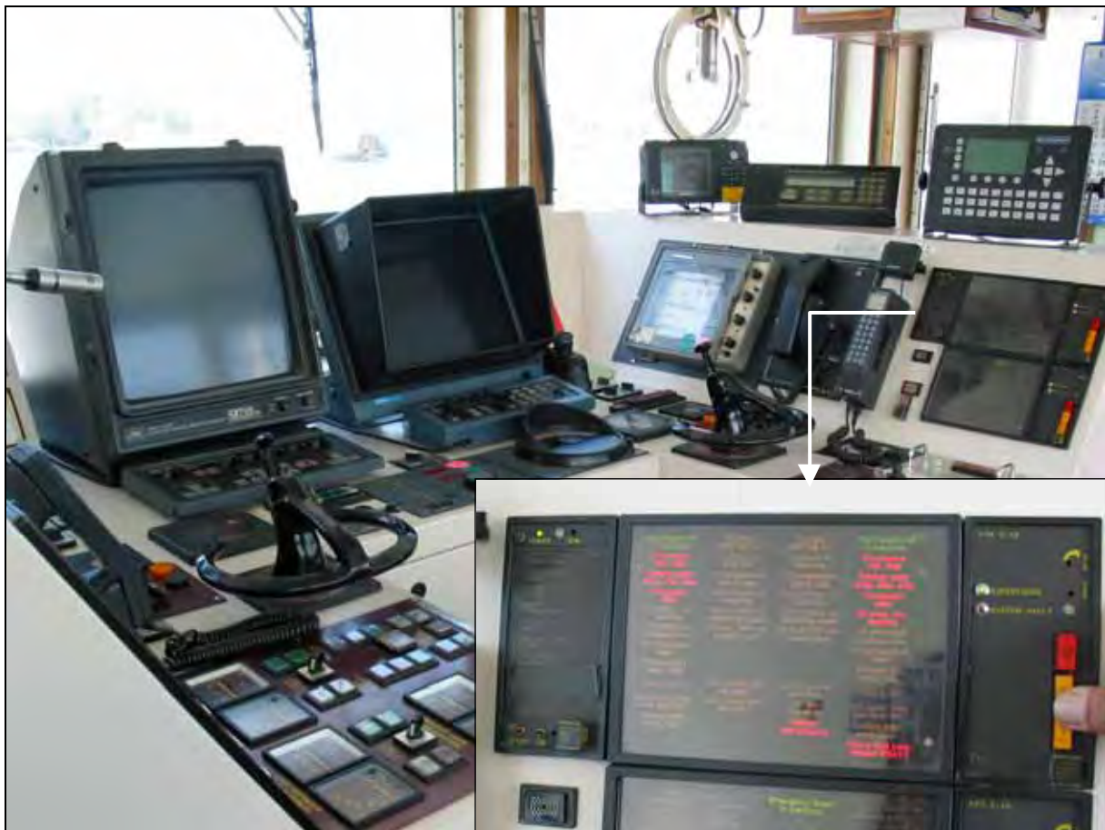
Figure 20: Alarm panel on the LASS URANUS' conning position
