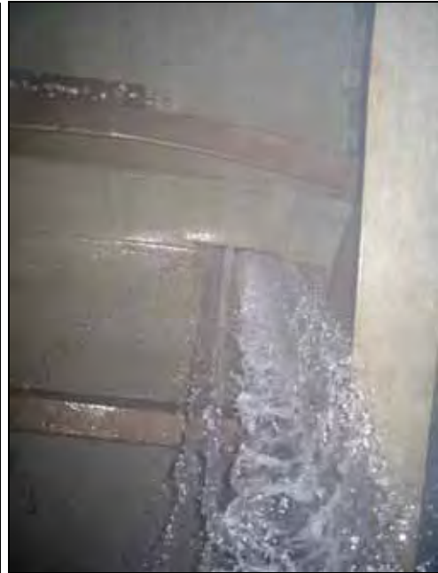
Figure 15: Tear in deep tank no. 1
