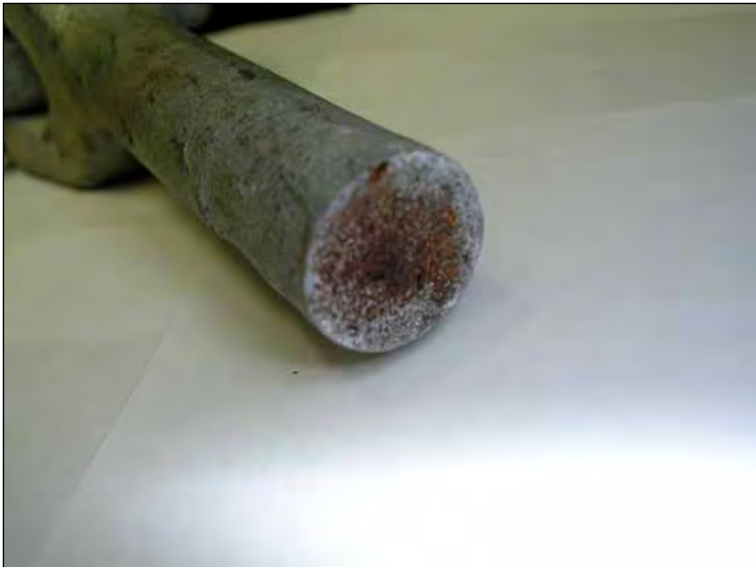
Figure 43: Corroded fracture surface of the lashing bar
