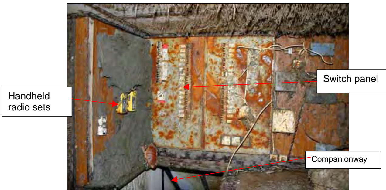
Figure 19: Companion-way and distress radio equipment
