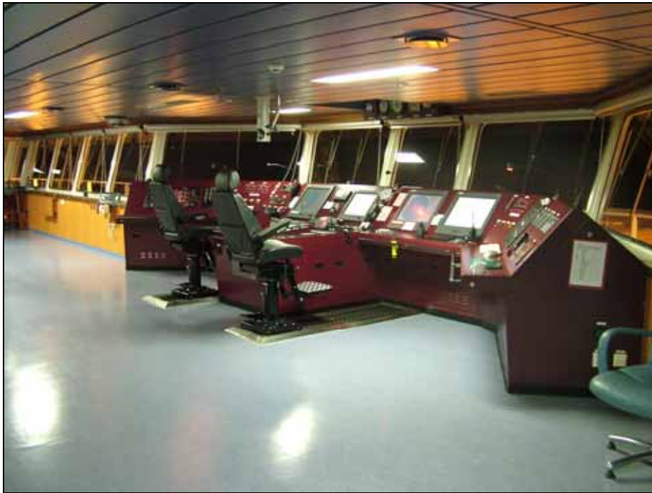
Figure 10: Arrangement of the bridge consoles on the LT CORTESIA
