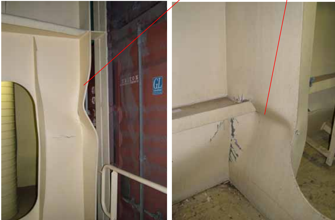
Figure 5: Damage to the frame bulkhead
