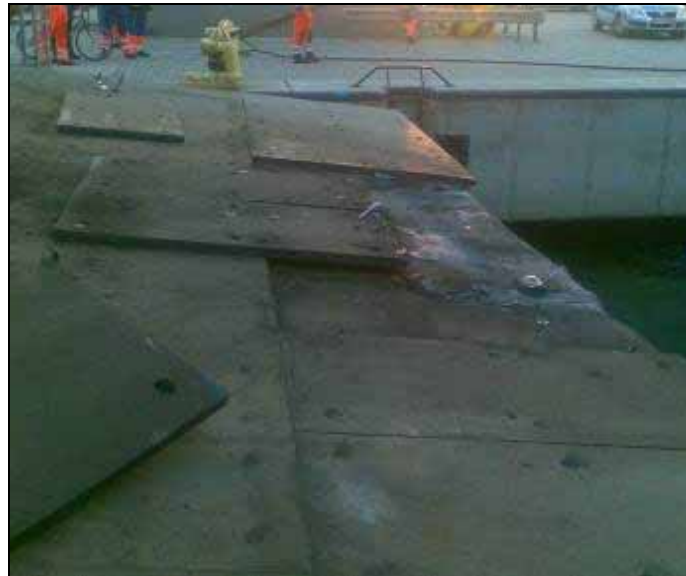
Figure 9: Damaged plating on the loading bridge
