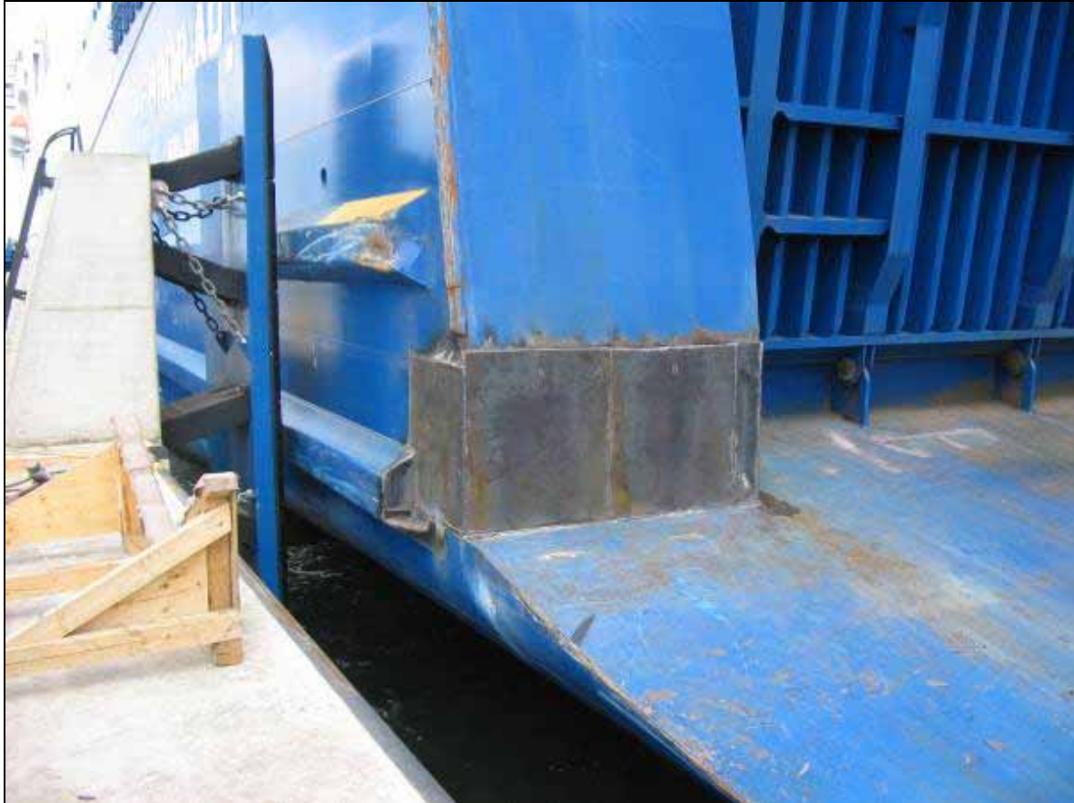
Figure 11: Emergency repairs to the damaged cofferdam
