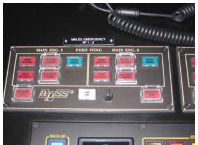
Fig. 4: Bridge wing conning station - emergency panel ME 1 and ME 2
