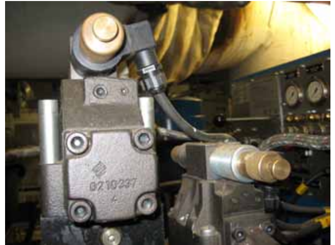
Fig. 14: Emergency operating devices - solenoid valves
