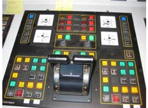
Fig. 10: Main propulsion monitoring panel (overview) - ECR
