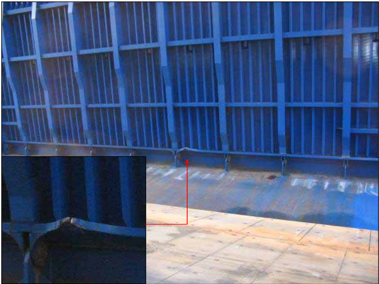
Figure 5: Damage to the stern ramp of the FINNLADY
