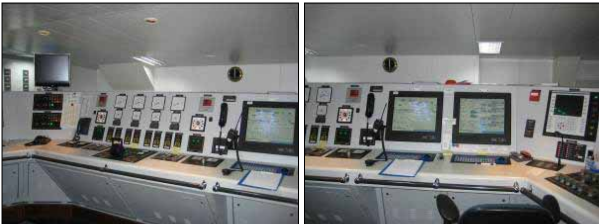
Figure 35: Drive and monitoring panel in the engine control room
