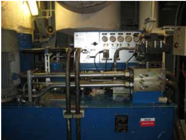
Fig. 13: CPP hydraulic-power pack with emergency operating devices
