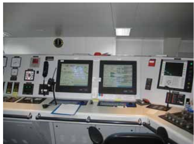
Fig. 12: Alarm monitoring console - ECR
