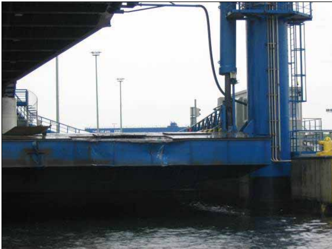
Figure 10: Damage to the steel substructure of the loading bridge
