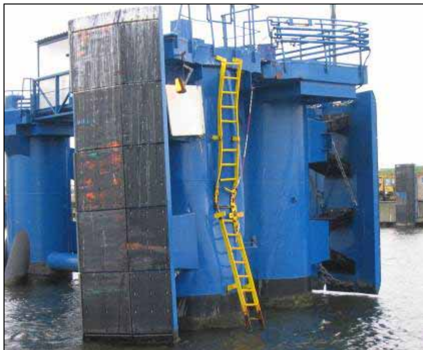
Figure 8: Damage to the foremost fender pile
