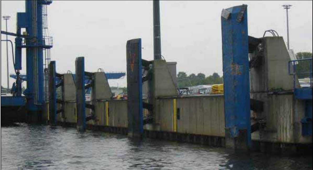
Figure 7: Damage to the fender piles
