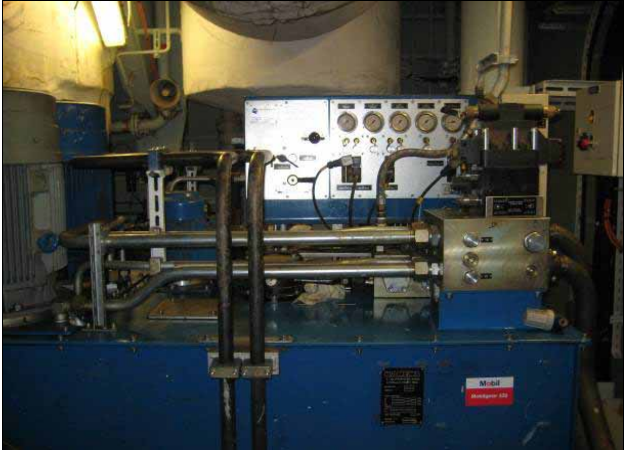
Figure 36: Hydraulic valve block
