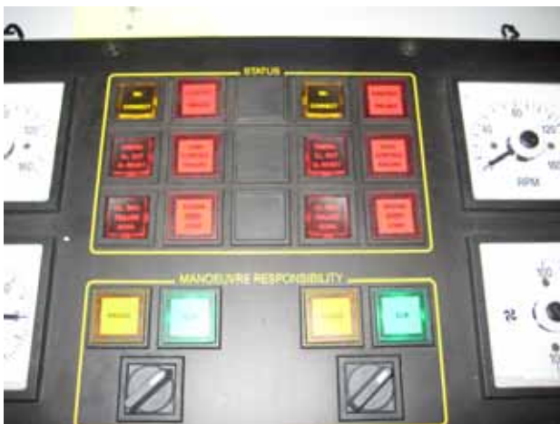
Fig. 11: Main propulsion monitoring panel (details) - ECR
