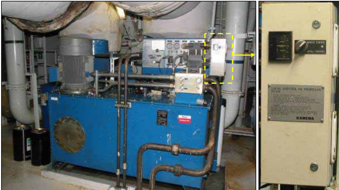
Figure 22: CPP unit in the engine room
