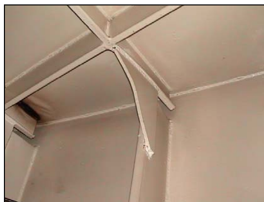
Figure 6: Deformation of the frames on the RABA
