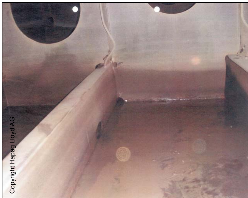
Figure 5: Bottom damage with deformations
