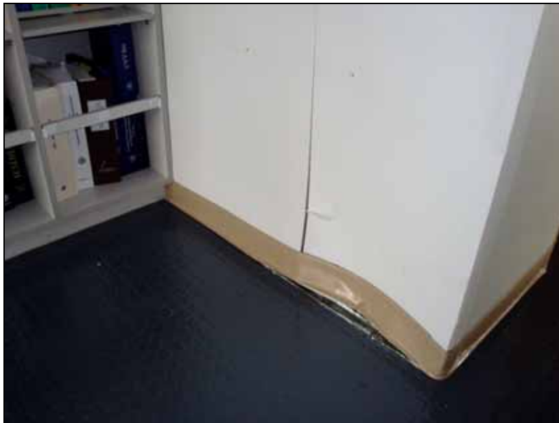
Figure 7: Deformed interior panelling at floor level 17
