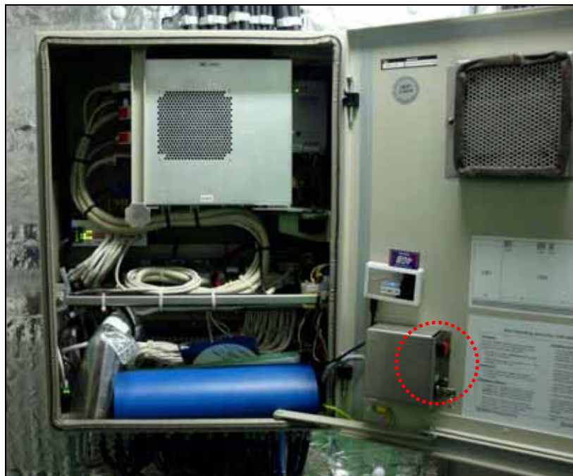
Figure 41: Switch for incident backup in the Main Unit
