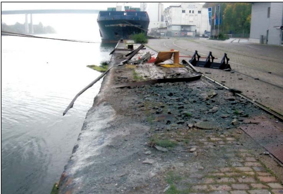
Figure 6: Damage to the pier
