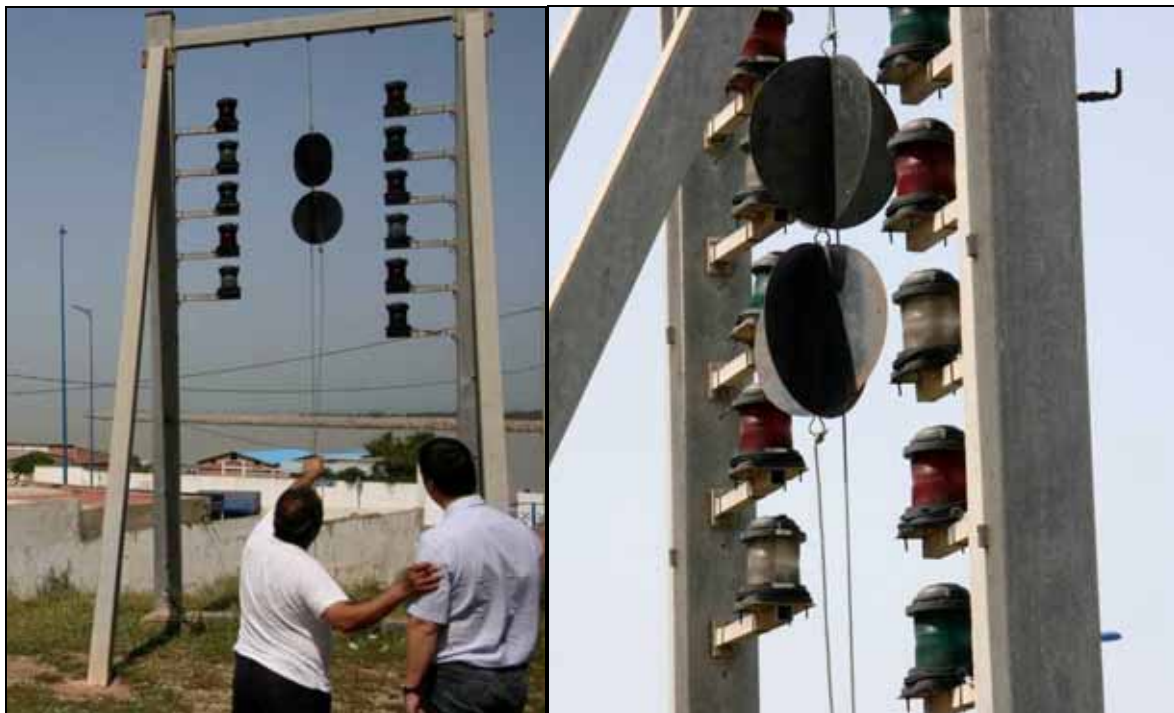
Figure 33: Port signalling system, details
