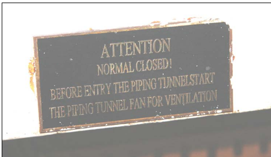
Figure 17: Notice plate above the pipe tunnel cover
