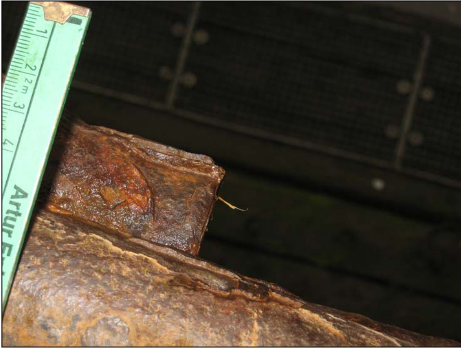
Figure 7: Strand of fibre on damaged element
