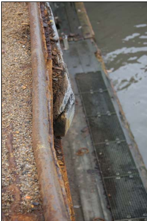
Figure 19: Damage in March 2010
