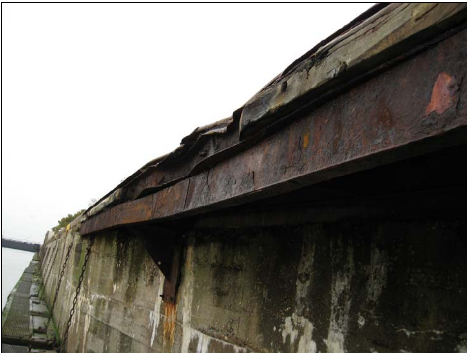
Figure 8: Damage seen from below
