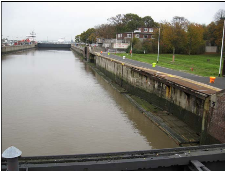
Figure 24: View from the outer wall with bollards, middle gate and safety recess
