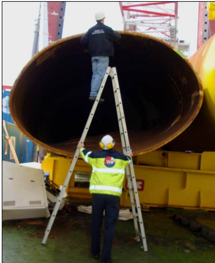
Figure 18: Inspection of the pressure marks 34
