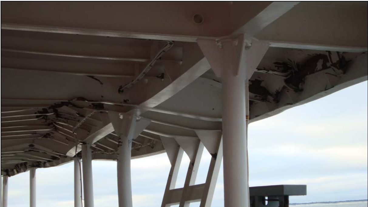
Figure 9: Damage photo 5 – CLEANTEC
