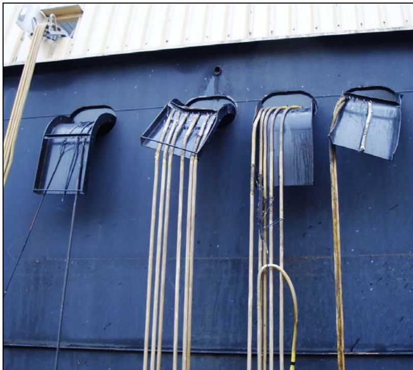
Figure 21: Damage to the shore connection points (3)
