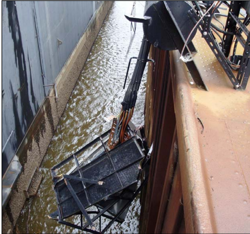
Figure 20: Damage to the shore connection points (2)
