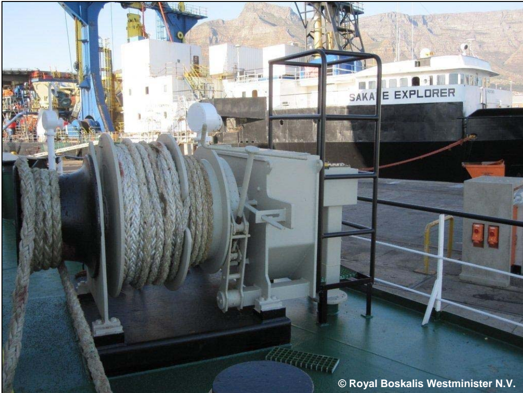
Figure 13: New position of the control unit of the winch with safety cage (1)
