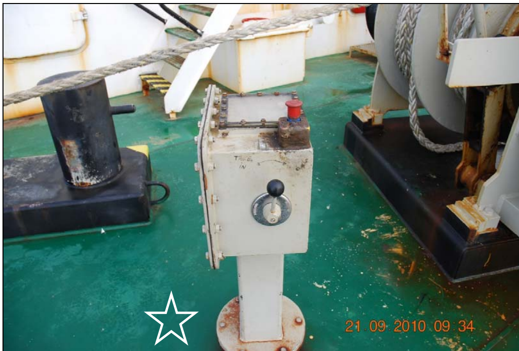
Figure 5: Close-up of the starboard winch's control station
