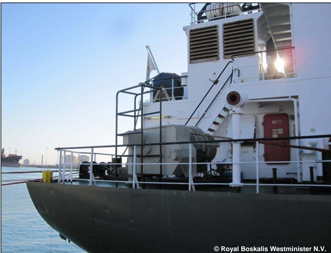
Figure 14: New position of the control unit of the winch with safety cage (2)
